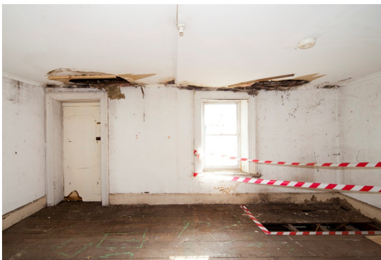
Figure 198. 48 Kensington Street This terrace is highly intact, with the only evidence of change to the fabric caused by the damage from water entering the building. The extent of damage suggests that there were significant structural leaks for many years. (photo Nat Hughes)
