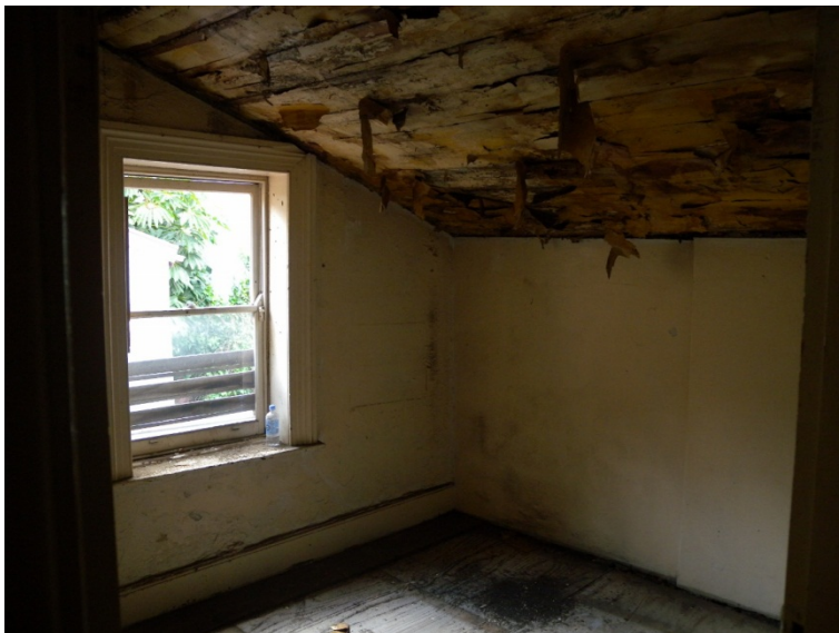
Figure 197. 48 Kensington Street Upper level – rear room under the skillion roof. The original timber/bark lining is in poor condition.
