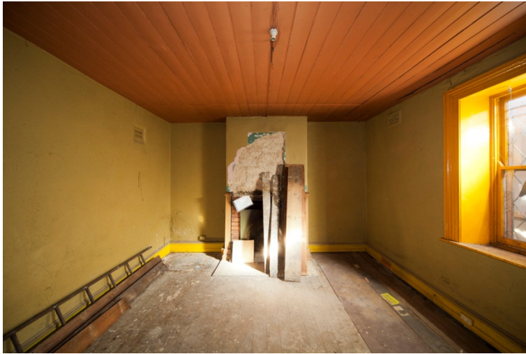
Figure 189. 46 Kensington Street. Main ground floor room. The mantle has been damaged by a fire in the grate (the working status of the chimney is not known) (photo Nat Hughes)
