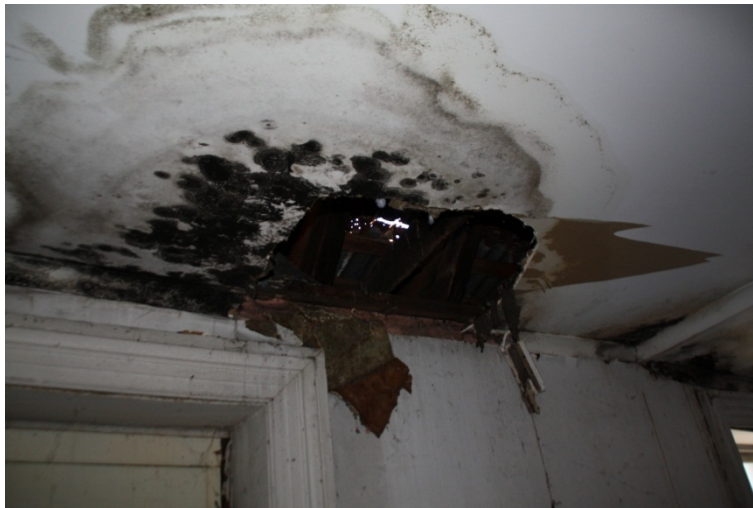
Figure 199. 48 Kensington Street Serious ceiling damage caused by water entering the roof space.
