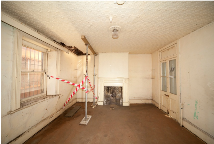
Figure 193. 48 Kensington Street Main front room. 48 is highly intact, although has suffered serious damage from water entry over many years. (looking north to the common wall with 46 Kensington Street). (Photo Nat Hughes)
