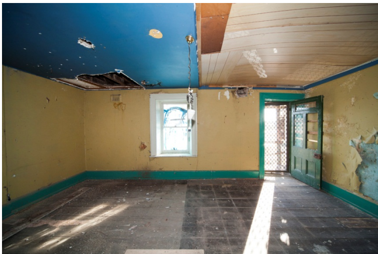
Figure 185. 46 Kensington Street. First floor main front room. Note original joinery and evidence of damage to ceilings being covered by lightweight boarding. (photo Nat Hughes)
