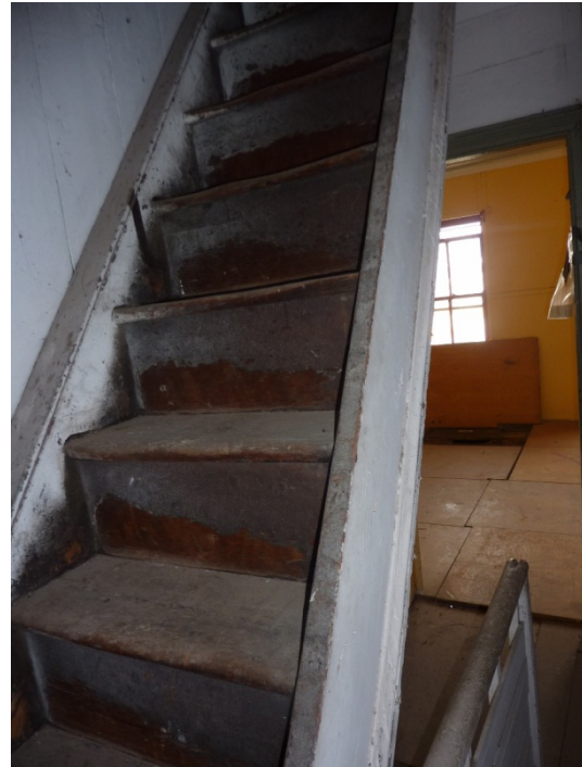
Figure 166. The stairs from the upper level to the former attic room are similarly pitched and do not have a handrail.
