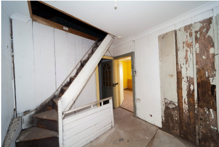
Figure 161. The stair continues from the first floor. Note the termite damage to the wide timber wall panels. (photo Nat Hughes)
