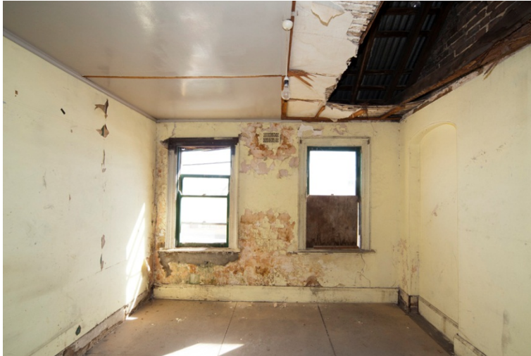
Figure 151. 36 Kensington Street Upstairs bedroom. Note deterioration to ceiling and evidence of water penetration to the front wall near the windows.
