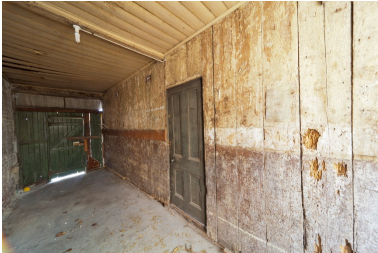
Figure 155. Carriage drive-through the building: The northern wall of the passage carriage passage retains its original wide vertical timber slabs (termite damaged). Ceiling is timber tongue and groove boarding. A timber 4-panel door provides direct access to the dwelling. (photo Nat Hughes)
