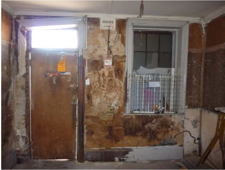
Figure 145. 36 Kensington Street. The street wall shows evidence of significant deterioration, although elements such as the original sash window joinery, have survived. (Photo: Nat Hughes)
