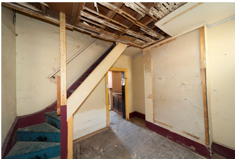
Figure 141. 34 Kensington Street Back (dining) room. This room is in more original condition, with significant damage to the lath and plaster ceilings and other elements. (Photo: Nat Hughes)
