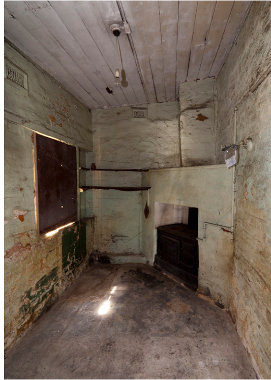
Figure 120. No.28: The original cooking range has also survived in the fireplace. Wall finishes are peeling, but the underlying layers of paint can be readily read and interpreted. (Photo Nat Hughes)
