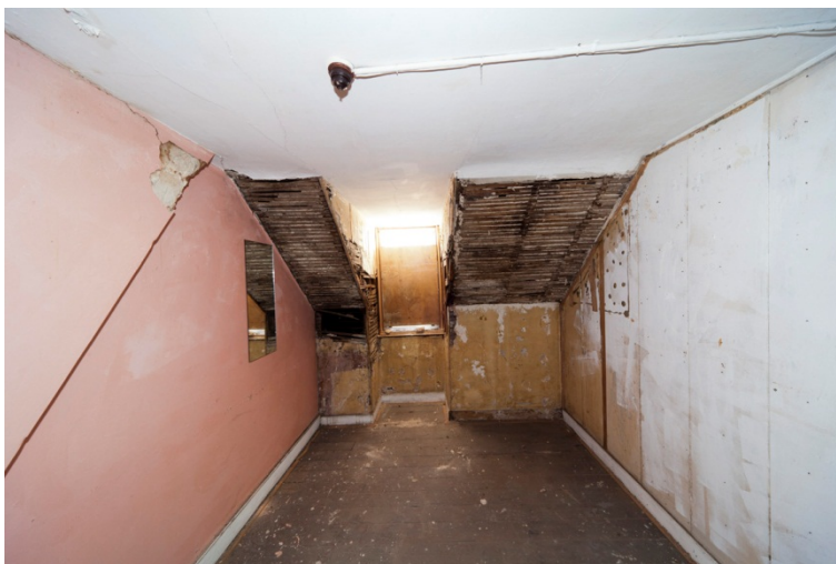
Figure 118. No.28: Attic room showing its original configuration. The plaster to the underside of the main roof plane has been removed/deteriorated. (Photo Nat Hughes)
