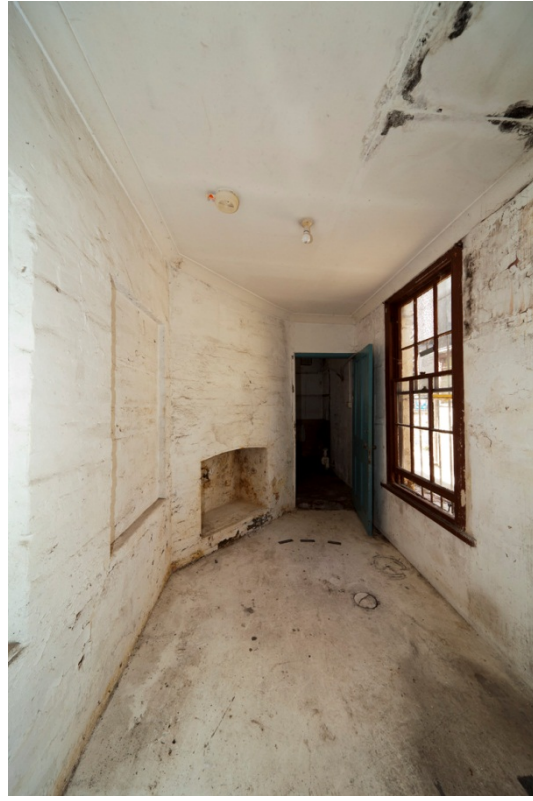
Figure 114. No.26 The original kitchen space has been stripped but its fabric is intact. Note water damage to ceiling panels. (Photo Nat Hughes)
