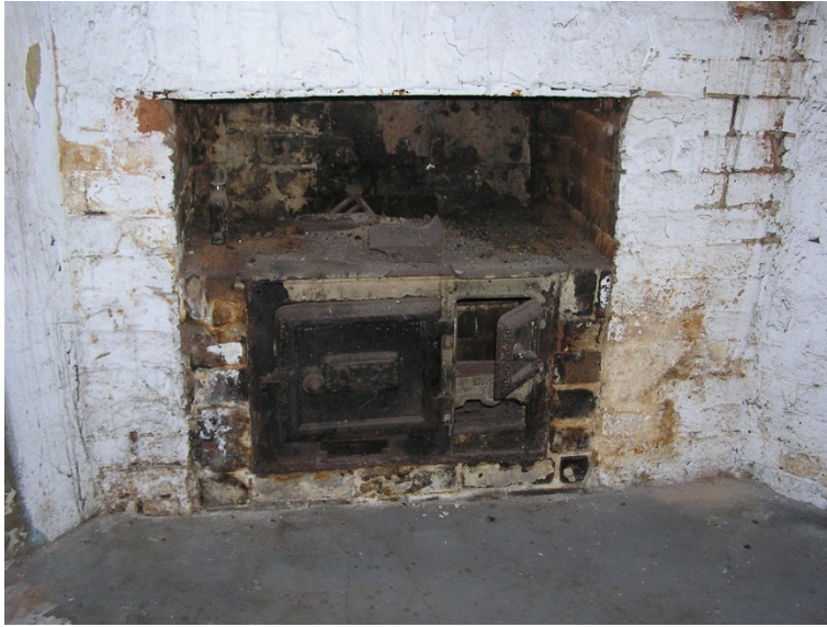
Figure 103. No.22: kitchen fireplace
