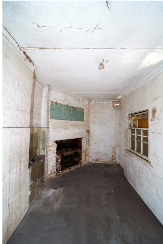
Figure 101. No.22: original kitchen area is intact but in poor condition.
