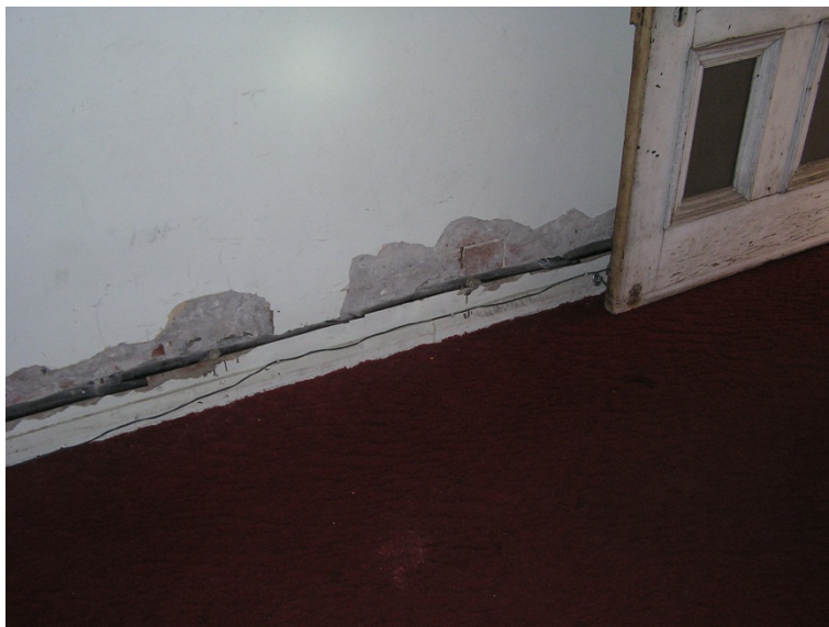
Figure 90. More recent damp proof course was inserted very crudely with significant damage to the original fabric (prior to the current ownership of the site).
