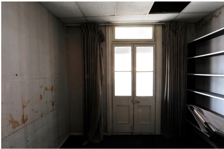
Figure 84. The fabric of the upper level has been similarly altered to provide late 20th century office space, although the arrangement of rooms is more consistent with the original. The fabric is showing signs of significant neglect and poor quality building work in the past.
