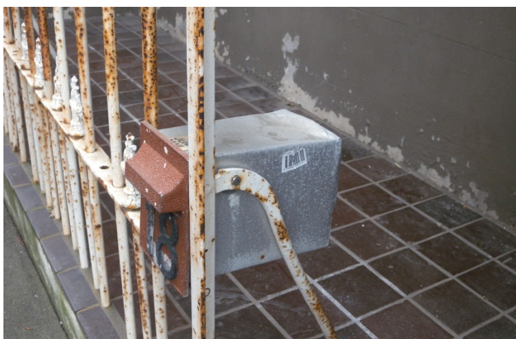
Figure 82. The floor to the veranda has been covered by glazed ceramic tiles. This has led to damage to the fabric of the walls due to the impermeable nature of the tiles.
