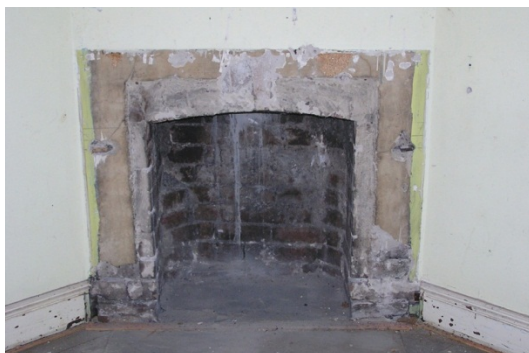
Figure 78. Internally, the terraces are reasonably intact although in poor condition: all extant joinery is original except the front doors. Ceilings are either damaged or not original, mantelpieces are either missing or not original. Much of the original joinery such as skirtings are intact.
