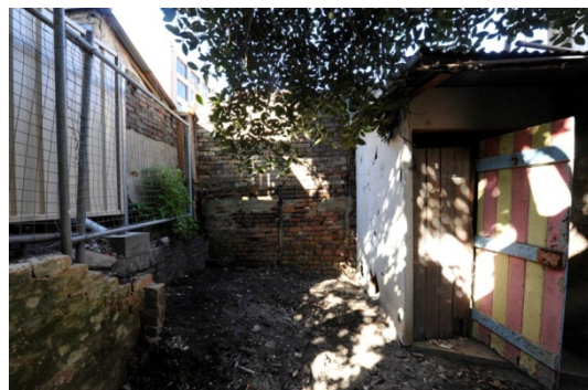
Figure 79. The rear yard was also found to be in very poor condition. It retains remnants of the early separate WC's, recently collapsed due to the actions of the developer of the adjacent site, elements of early side walls that are now incorporated into other construction, small areas of remnant pavements, several large trees and a de-stabilised rear property wall with some new retaining wall construction related to adjacent properties.
