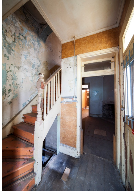
Figure 73. The stair to 16A remains trafficable (Photo: Nat Hughes)
