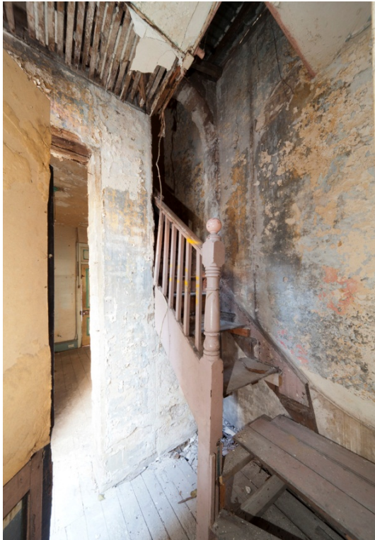
Figure 72. The stair to 16 is in very poor condition (Photo: Nat Hughes)
