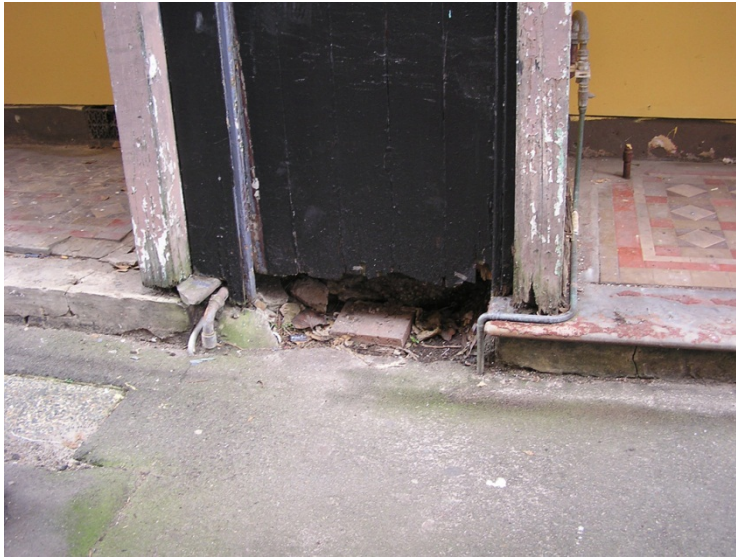
Figure 67. The fabric is original, but showing signs of deterioration.
