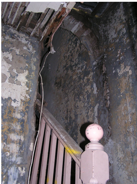
Figure 76. Stair to No.16 showing poor condition.
