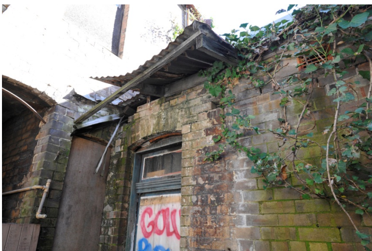
Figure 69. Detail of deterioration of the roof iron and brickwork to the skillion wings to the rear of the main building.
