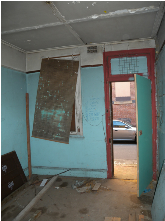
Figure 74. Main room to No. 16. The rooms are small, and although the spaces are intact, much of the fabric is in poor condition.
