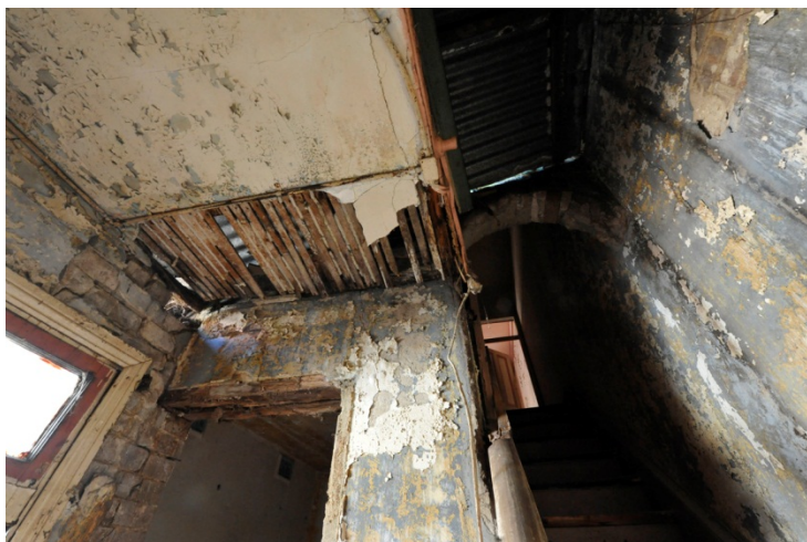
Figure 71. Roofs are corrugated steel. Roof flashings have failed and allowed water into the buildings causing a range of structural issues and failing interior and exterior finishes. (16)
