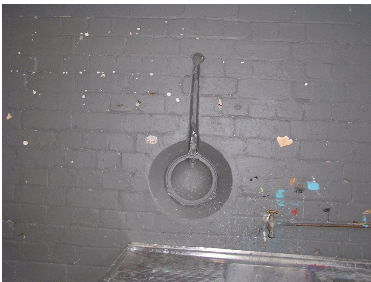
Figure 45. Fittings for safety lights have survived throughout the building with raw wiring to the ground floor in administrative area.
