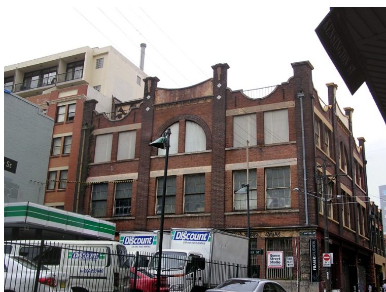
Figure 27. The parapet is formed of brick with cement capping and a cement render finish to the rear (roof side). The parapet has been braced on the roof side but is deformed in places. Inset iron grille rails to the scalloped profile of the parapet are rusting and their soundness is not known. The roof is a simple gabled structure set behind the parapet and is clad in corrugated iron sheets. Some sheets have surface rusting in places but they appear to be relatively new and generally sound: inspection of the interior of the roof space revealed few holes and no evidence of recent water ingress. Flashing has been replaced where the roof abuts the parapet – there is evidence of earlier water damage to the brickwork. The old flashing sheets are stored within the roof space.
