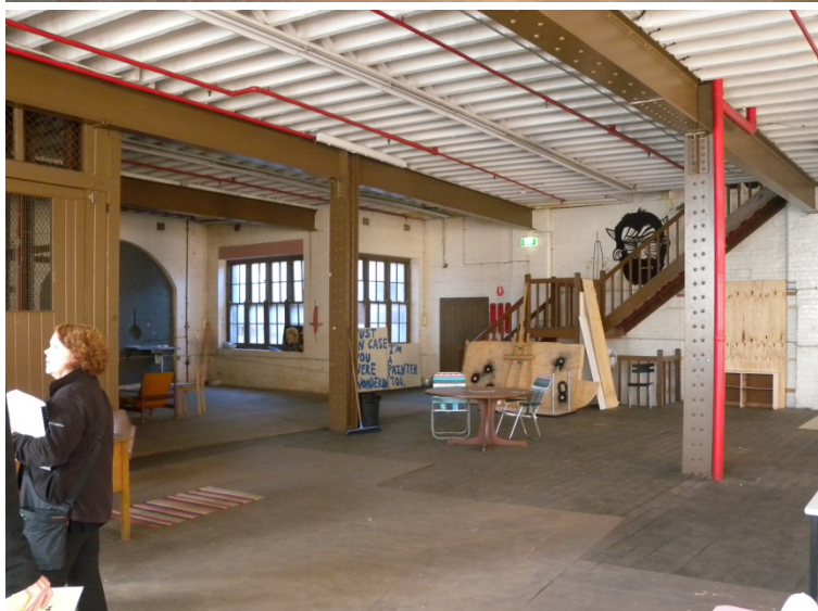
Figure 35. Level 1 – Similar to the ground level, – same structural configuration including riveted beams and columns. Floor-ceiling heights are less than the other levels. Some cracking to wall at top of the light well due to water ingress. Ceilings throughout are open to the undersides of the timber joists and floorboards of floor above with herringbone bracing..
