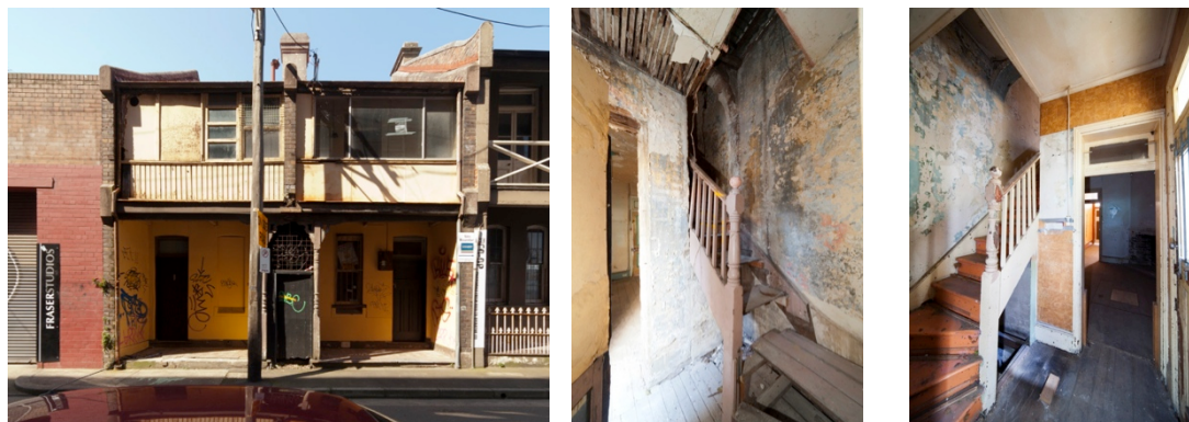
Figure 8. Terraces at 16-16A Kensington Street (1906). Both are substantially intact. No.16 is in poor condition with significant damage to the structure and building elements and 16A is in poor to fair condition. Both require extensive repairs to be habitable. (Photos Nat Hughes)
