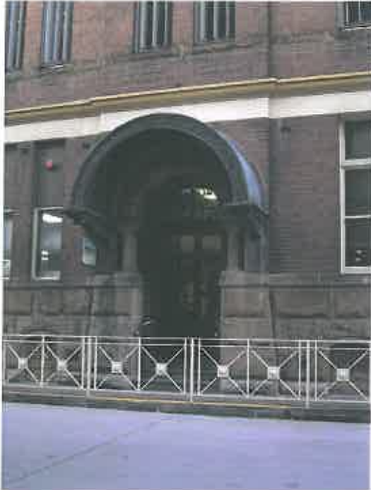
Figure 36 - Exterior view of the main entry door to the Administration building 10B showing the Romanesque entry doorway and cantilevered copper hood
