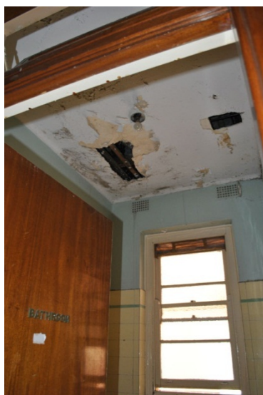
Figure 97 and 98. Bathroom areas. Evidence of water damage can be seen.
