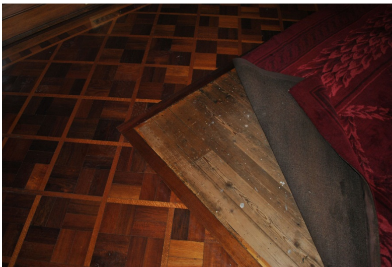
Figure 68. The parquetry, although visually rich, is limited to a band around the perimeter of the room, with the centre area (and concealed by the large carpet area) laid in simple unfinished floorboards.
