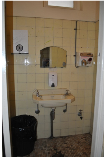
Figure 84. (left) Internal doors have retained their original deco lettering. Figure 85. (right) The bathroom areas on the ground floor are in original condition.
