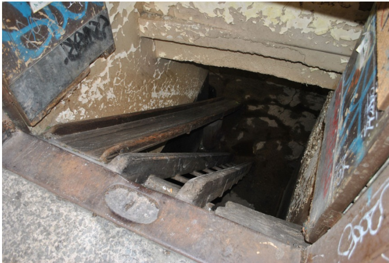
Figure 79. The robustly constructed timber keystone and case chute to the cellar has survived intact.
