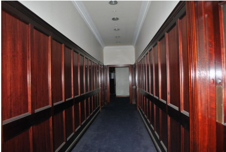
Figure 56. The panelling continues along the corridor to the Boardroom. A different timber has been used to that found elsewhere in the building, suggesting that it was installed at a different time.
