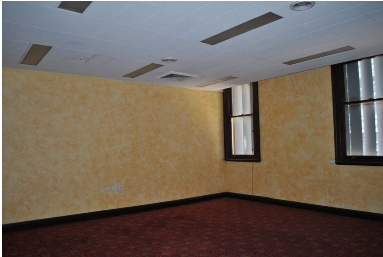
Figure 71. The former executive dining room has been refitted as a contemporary office space. It is not known whether panelling survives behind the contemporary finishes. Note also the adverse impact of the lowered ceilings relative to the sill height.
