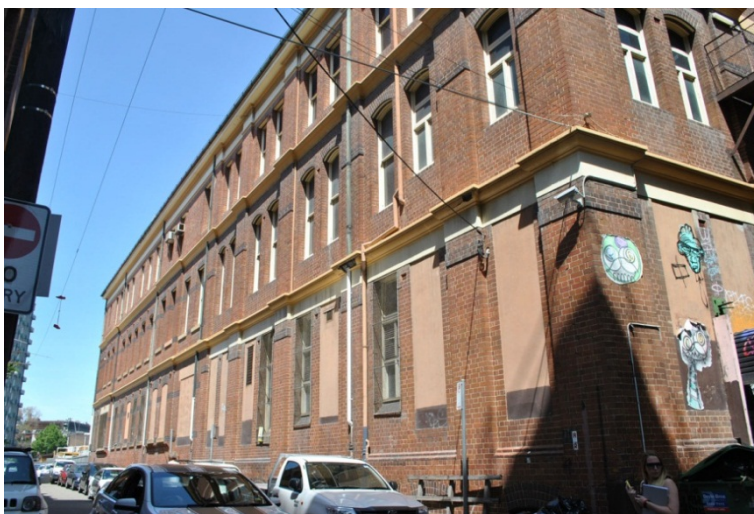
Figure 40. The condition of the external fabric appears to be generally sound, with the main areas of damage noted being limited to the PVC downpipes used to the lower levels of the building, and which have now cracked and broken allowing water penetration and some deterioration of brick jointing.
