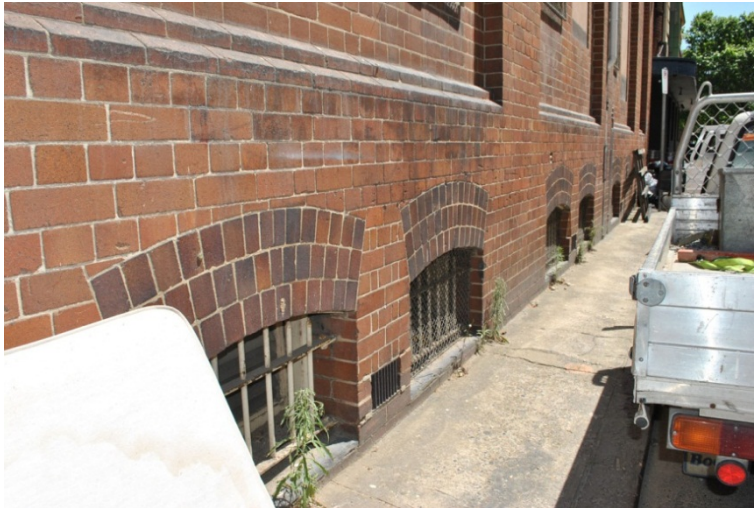
Figure 39. The 1930s extension provided gridded windows to the basement on Kensington Street.
