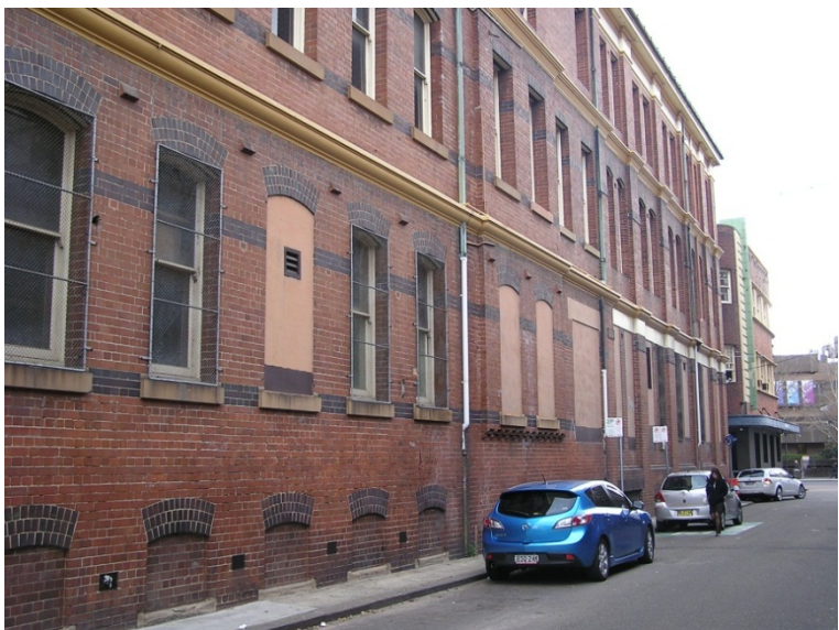
Figure 38. The building turns its back on the adjacent Kensington Street, with no door openings and groups of windows set high above the footpath level to allow light. The windows to the basement have been infilled with brickwork at the southern (1910) section and protected by utilitarian heavy grilles to the northern (below).
