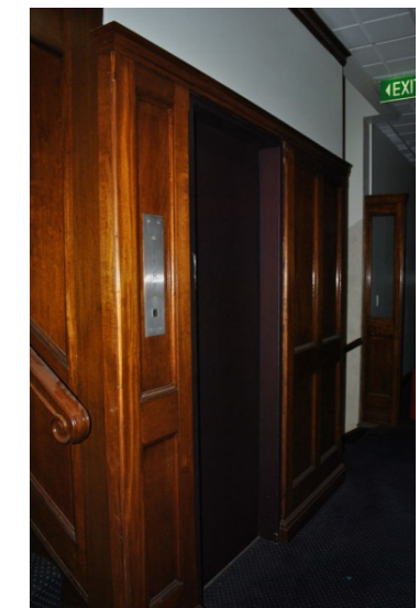
Figure 44. The stair to Level 1 is simple and not lined. It is likely, given its prominent position next to the access to the main lift that led to the Boardroom, that it was originally panelled.
