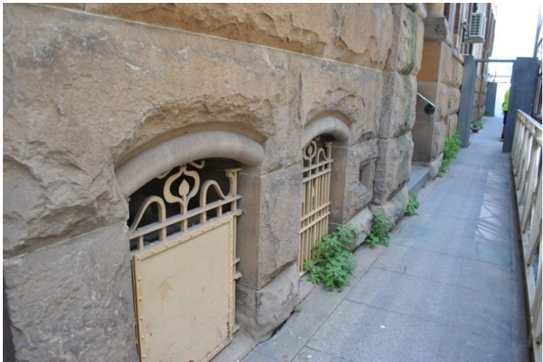
Figure 37. The Carlton Street elevation is set on a rusticated stone base into which the basement windows are set, the openings finished neatly with a dressed roll. The basement windows are protected by worked iron grilles in the Art Nouveau style.
