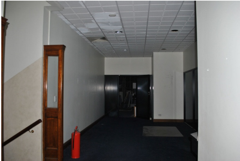
Figure 52. Looking to the south from the Level 1 vestibule. This area also reads as a late 20 th Century office space.
