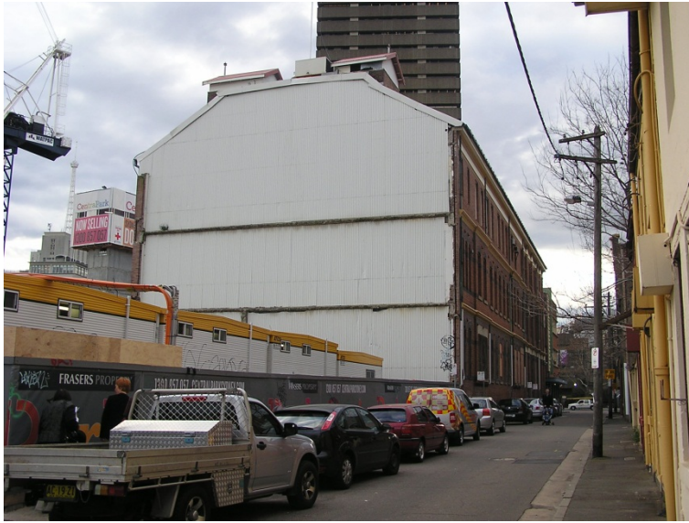
Figure 32. Southern elevation of the Administration Building showing the temporary wall erected to protect the Administration Building following the demolition of the earlier extension.
