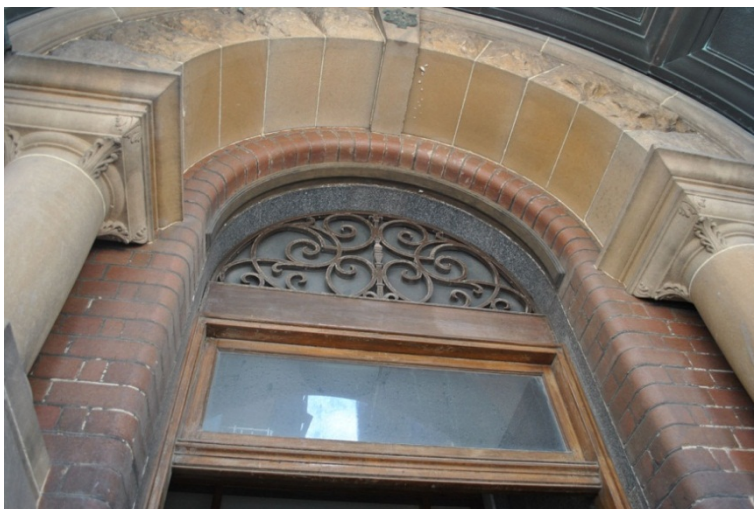
Figure 34. The formal entrance to the building is positioned at the centre of the western facade of the building and opens into the internal road. Protected by a simple Romanesque style arch and a copper hood, its restrained design and quality construction allow it to play an important part in the composition of the building.
