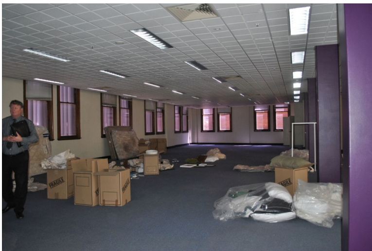
Figure 51. The main area of Level 1 has also been gutted and open plan office style fitout. Note the low ceilings created by the suspension of services under the timber ceilings which limit natural illumination and give the space a claustrophobic air.
