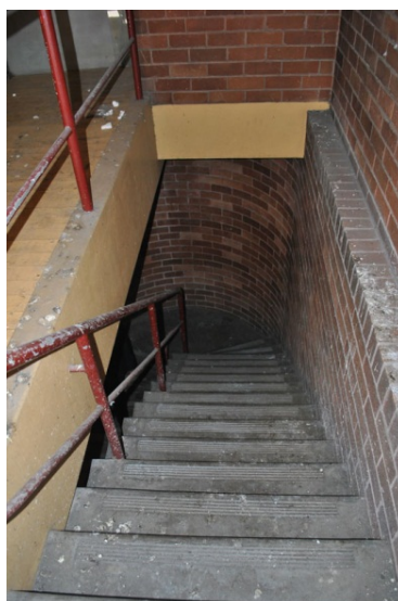
Figure 68. Looking into the lightwell from the roof terrace. This lightwell will be infilled to provide the supporting core for the levels above.
