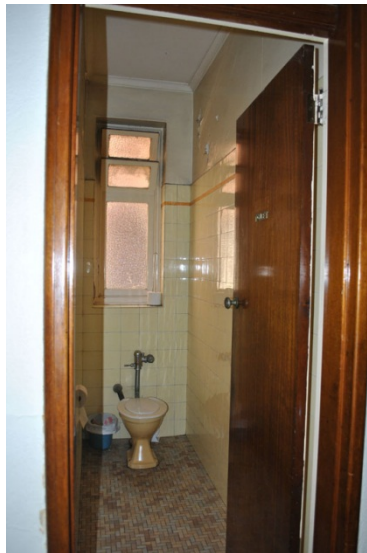
Figure 67. Existing bedroom and bathroom areas. These will be demolished and the area refitted for use as meeting rooms (Level 1) and restaurant (Level 2).
