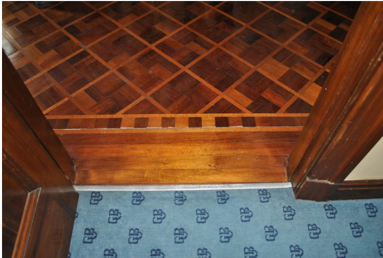
Figure 29. The floor to the Boardroom is richly laid parquet. This will be retained.
