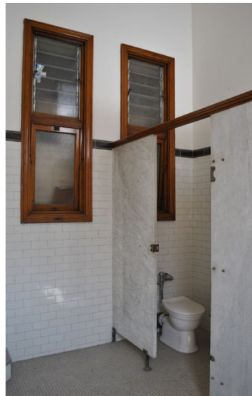
Figure 31. The executive washroom is intact. It will be retained with the insertion of an opening on its western wall to provide access to a separate bathroom area beyond.
