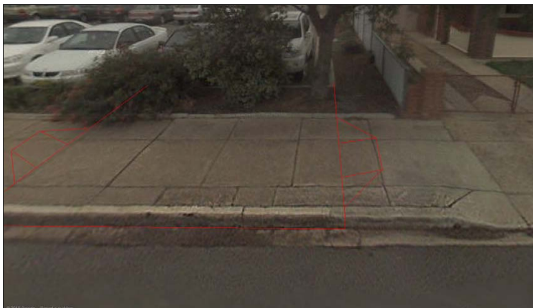
Figure 5.4.1 – Broken Kerb/ Footpath on Northern Side of Yabtree Street
