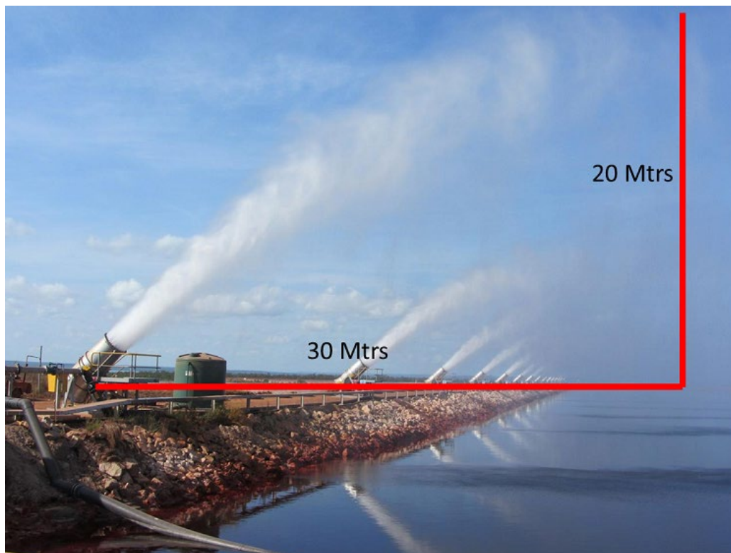
Figure 4: Example Spray from Evaporator Fan Operation (Minetek)
