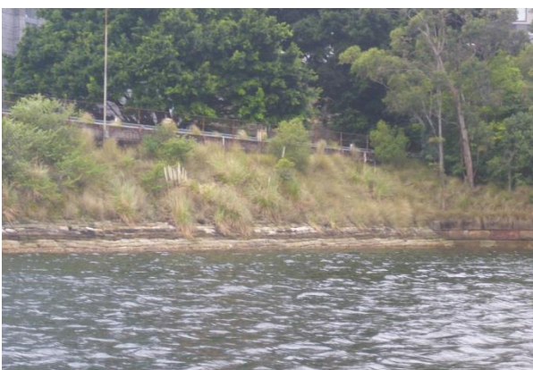
Picture 1 - Bridge embankment and stone sea wall (to the north of the subject site)
