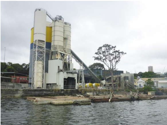
Picture 13 – Hymix concrete batching plant
