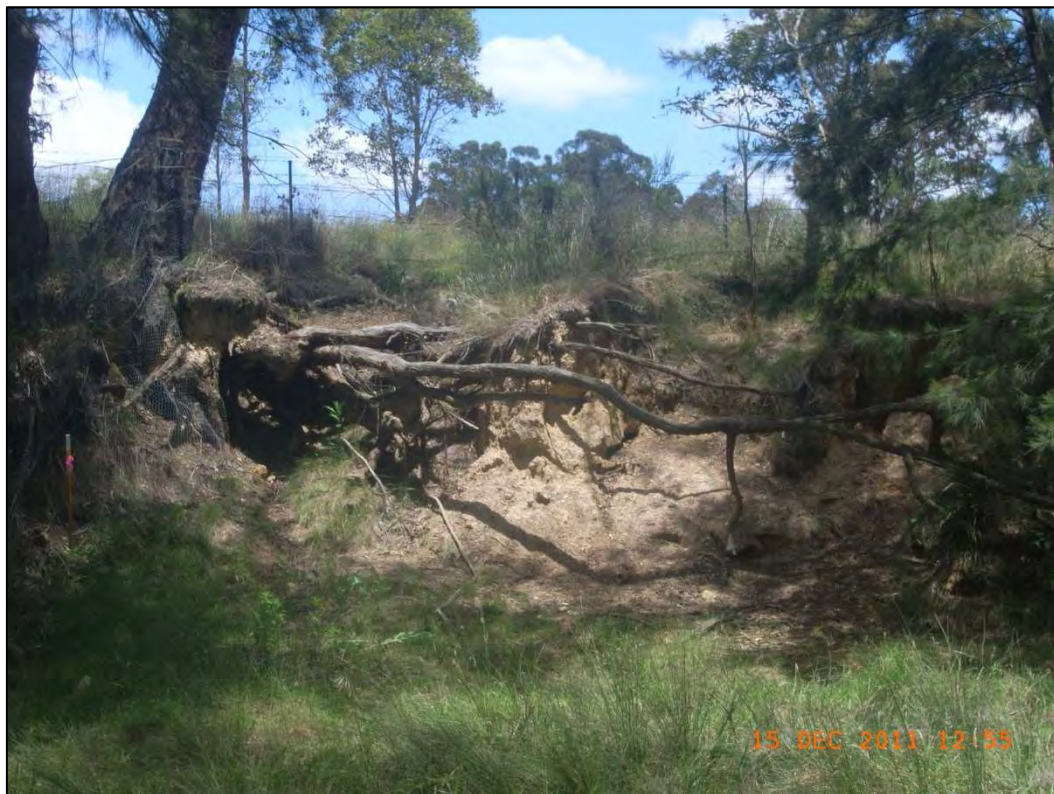
Figure 17 Right bank face. Exposed bank with active signs of erosion most likely a result of stock access to creek.
