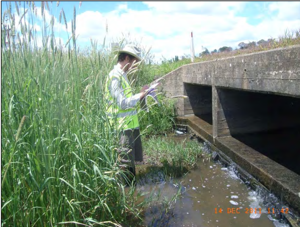
Figure 4: Downstream side of existing Ophir Road culvert. Small unnamed creek with a wide flowpath results in shallow flow depth. Well vegetated in-stream with grasses with silt and clay bed/bank material, no deep rooted vegetation or trees on banks.
