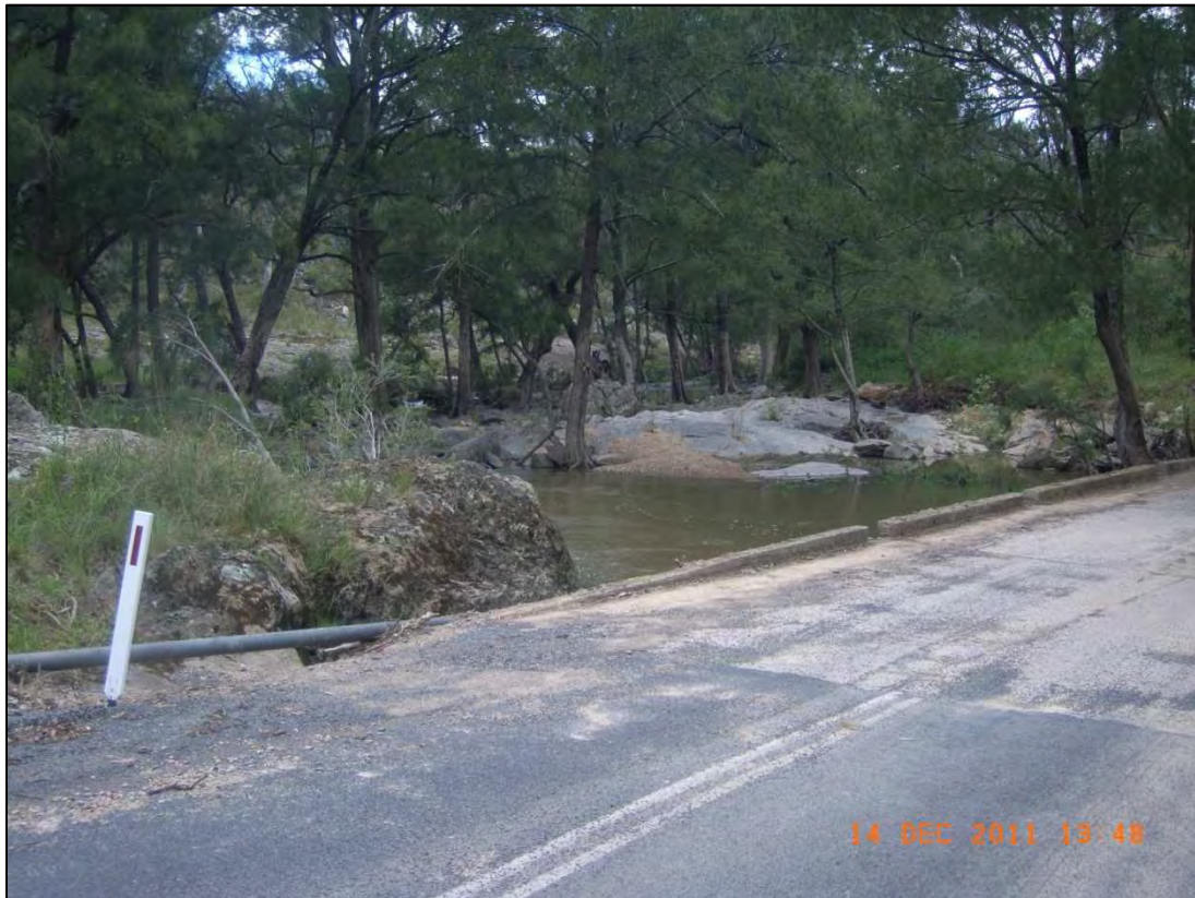
Figure 10: Looking downstream from Ophir Road. Creek channel controlled by bedrock with pockets of deposited gravel, silt and clay.
