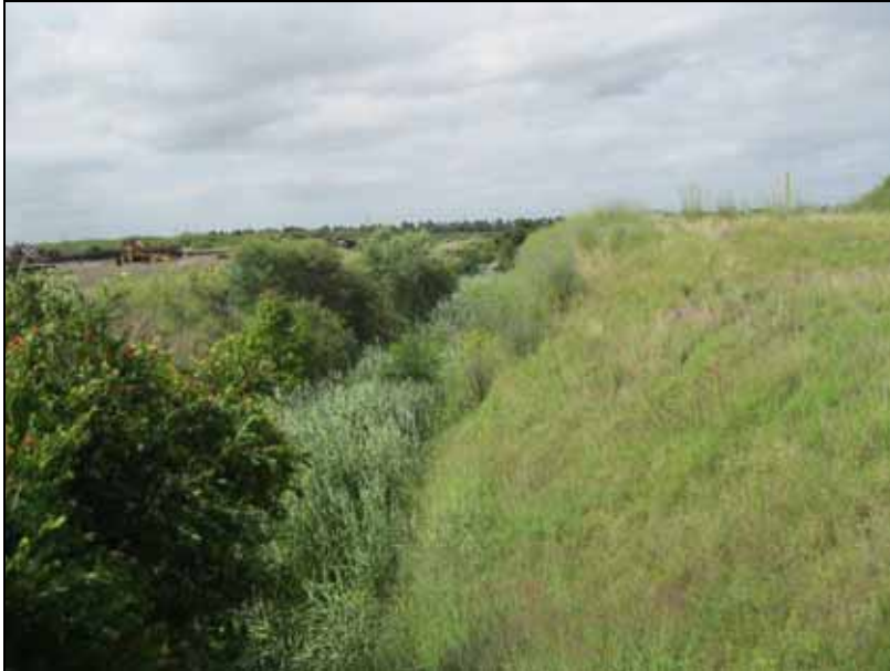
Figure 2: Open drain in the central portion of Site F, looking north (December 2011)
