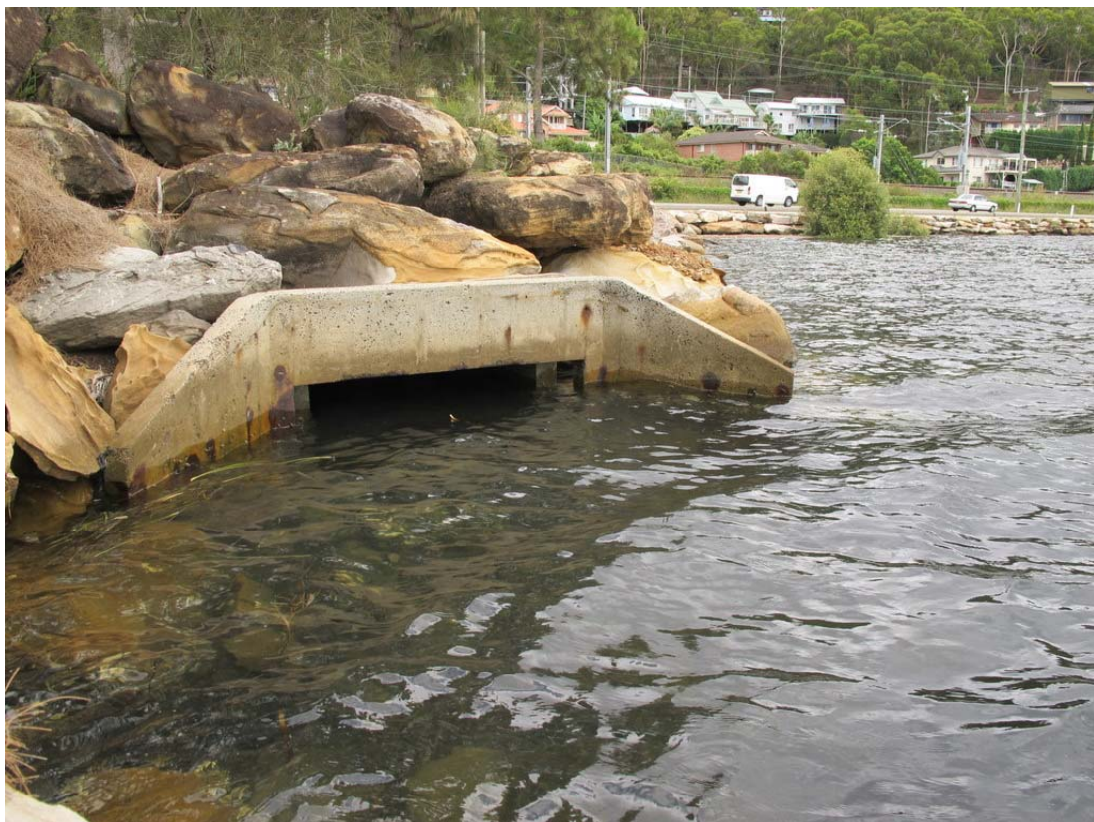
Plate 2: Upper: North-western stormwater drain seen at a low tide. Lower: High tide.
