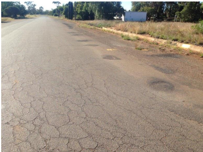
Cracking and deformation on the southern section of the intersection
