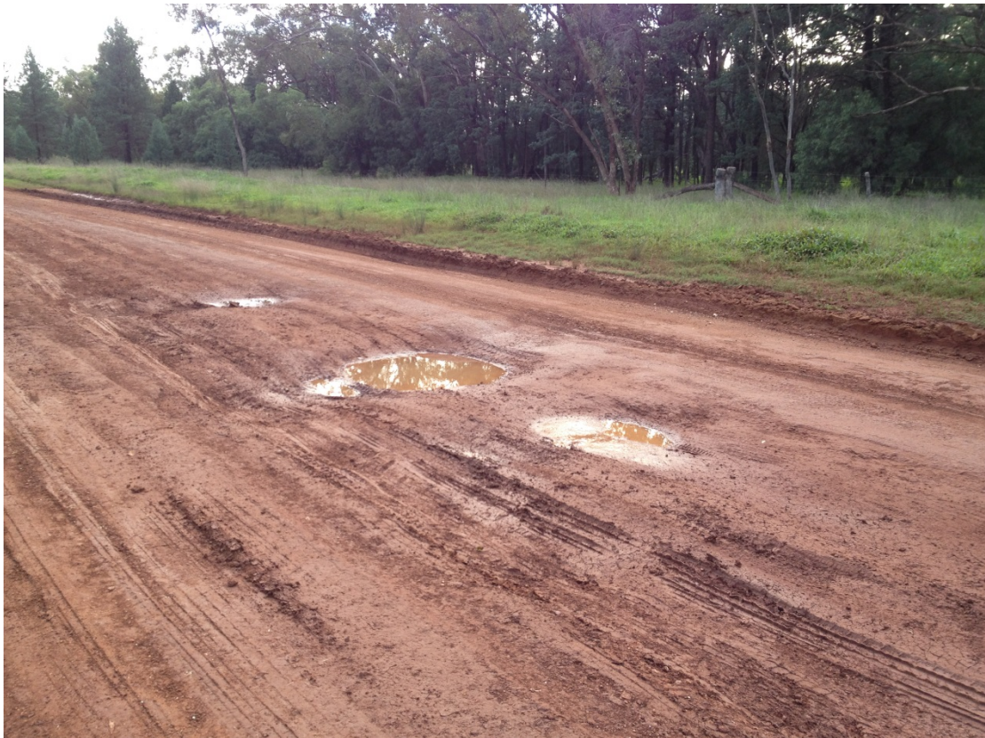
Plate 8: Nymagee-Hermidale Road gravel pavement section showing current poor condition.
