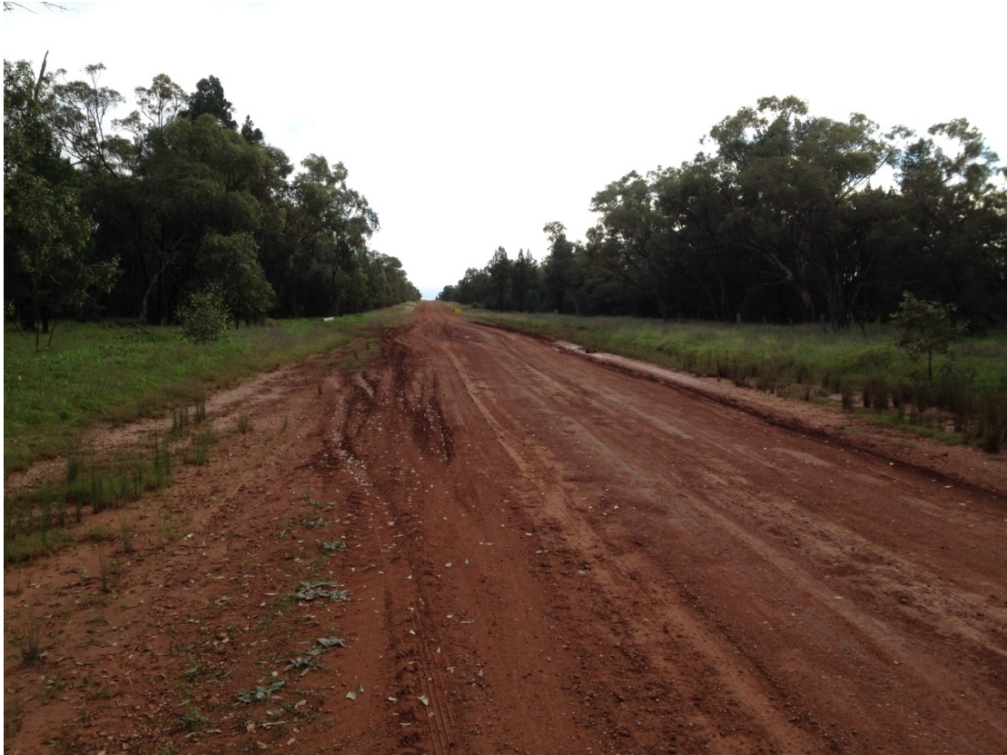
Plate 7: Nymagee-Hermidale Road gravel pavement section showing current poor condition.
