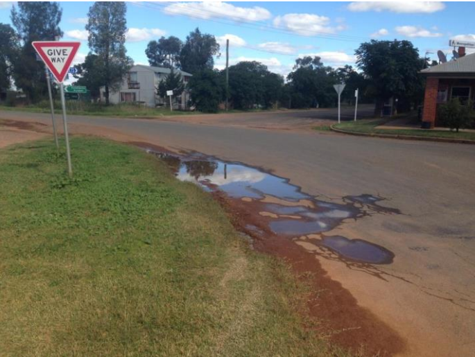
Water pooling at southeast section of the intersection
