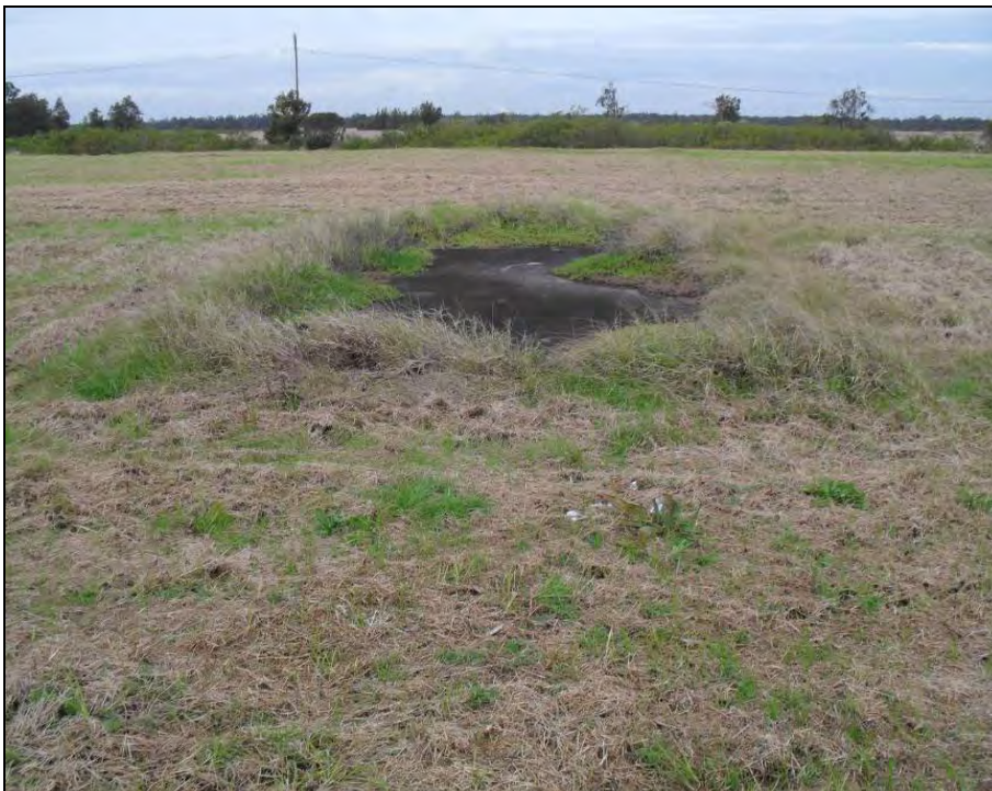
Photo 27 – Concrete slab in grassed paddock. Metal fragments/wire at surface of slab. (looking south)
