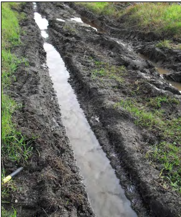
Photo 12 – Ash fill within track and possible hydrocarbon sheen at right edge of rutting
