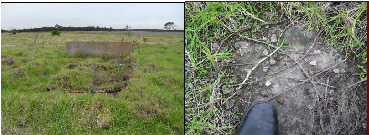
Photos 30 & 31 – Concrete slabs of former structure in south western corner of site. Fibro fragments, glass fragments, plastic, metal observed at ground surface.
