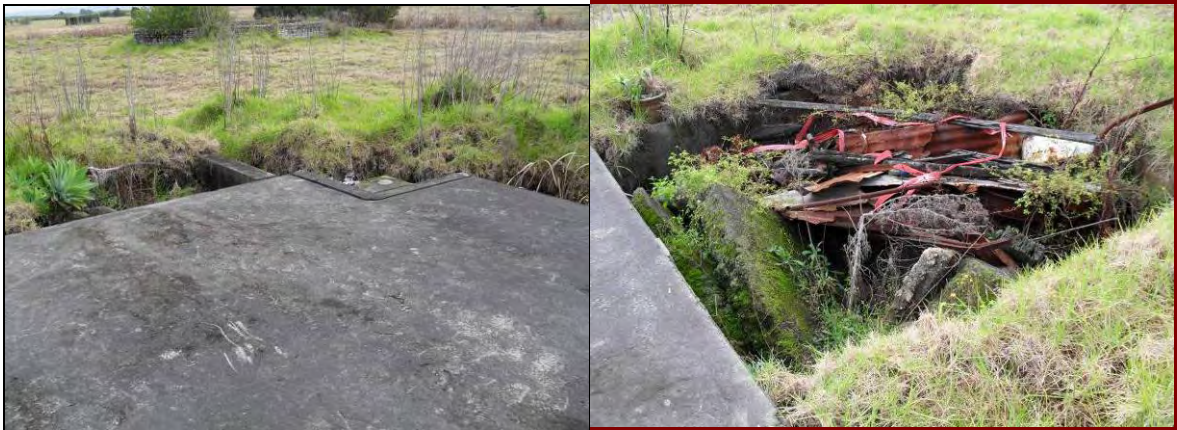
Photos 34 & 35 – Concrete lid of structure north of octagonal brick structures. Dumped demolition waste within sunken concrete chamber comprising scrap metal, concrete, metal sheeting, wire, timber, plastic, metal parts, possibly fibro cladding on walls.
