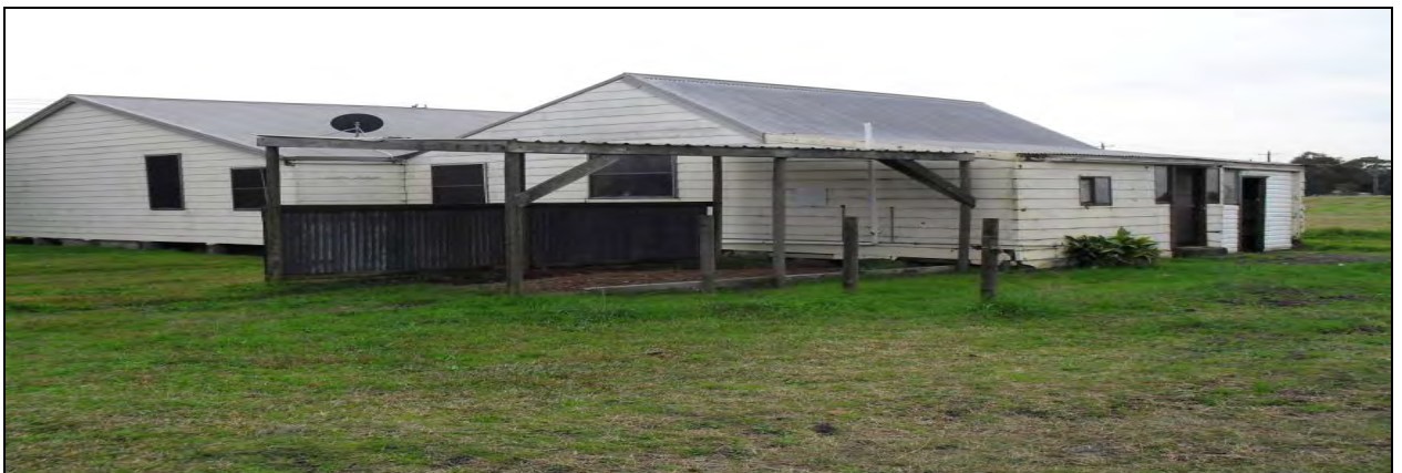
Photo 23 – Vacant dwelling and rear carport (looking north-east). Fibro sheeting observed in internal walls. Undulating ground around house (Possible fill).
