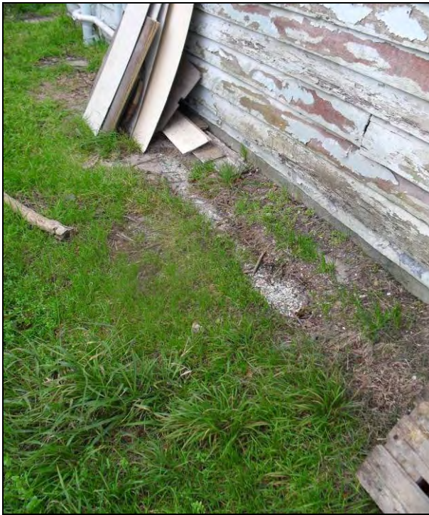
Photo 45 – paint flakes at ground surface adjacent dwelling
