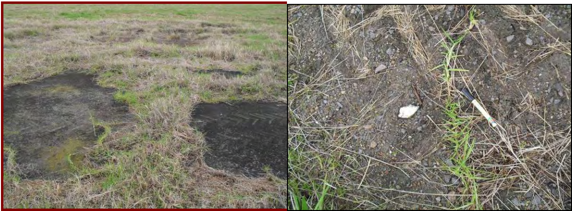
Photo 28 & 29– Concrete Slab in grassed paddock. Some asphalt pavement to south of slab. Some fibro fragments and gravel observed over slab surface.
