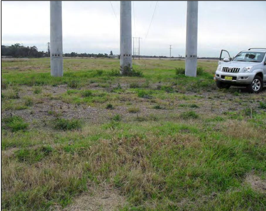
Photo 37 – Base of electrical transmission power poles in paddock. Granular fill pad comprising crushed rock and gravel at the surface around poles (looking north-east).
