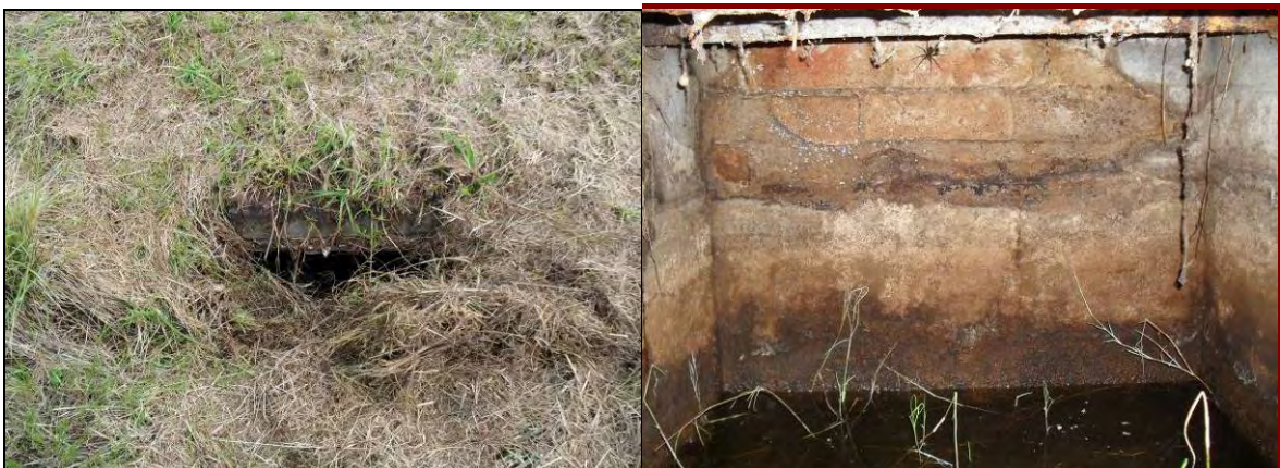
Photos 41 & 42 – Hidden brick, concrete and fibro sheeting clad septic chamber within grass paddock
