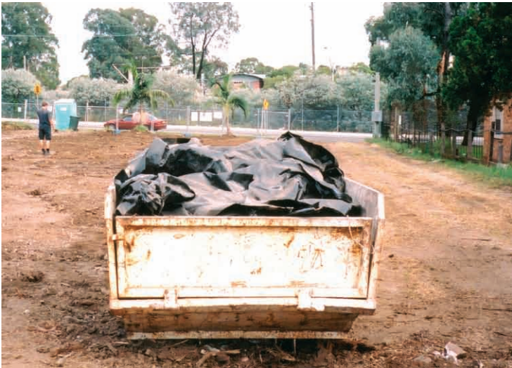
WRAPPED ASBESTOS WASTE
