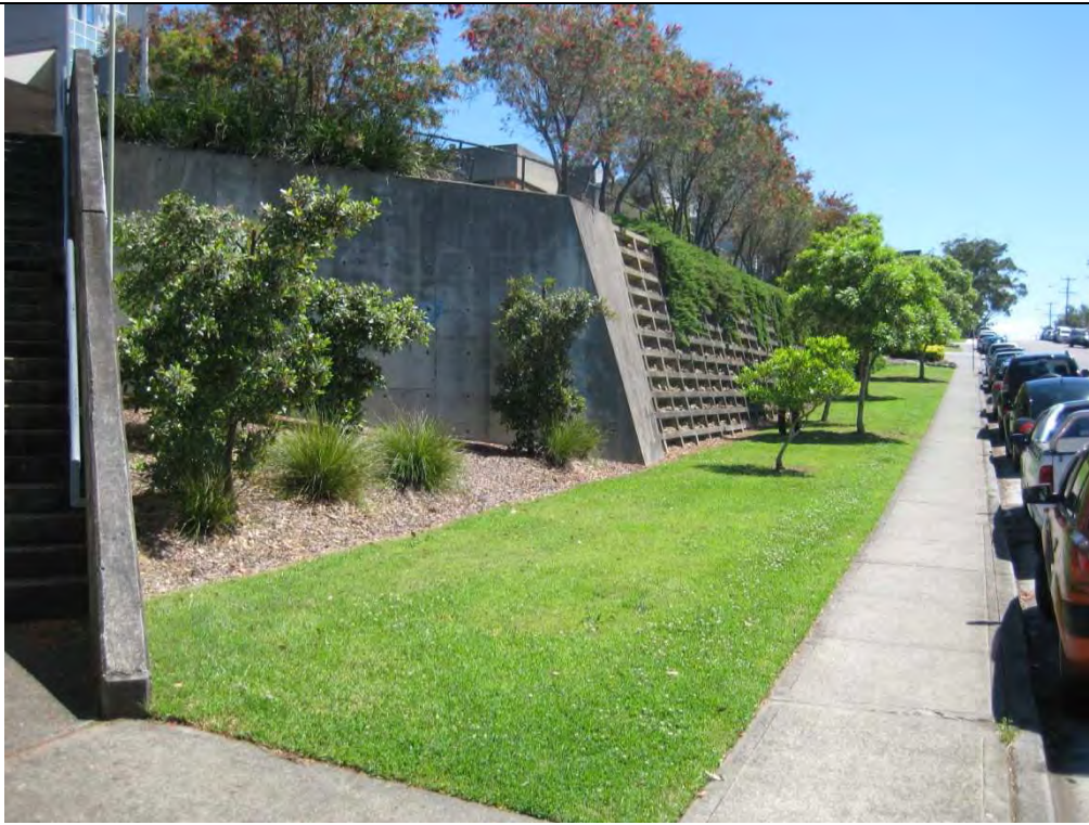
Photograph 1: Looking at the retaining wall along the eastern boundary of the site. The site is located at the top of the retaining wall. The height of the retaining wall varies from approximately 1m at the northern end to approximately 5m at the southern end
