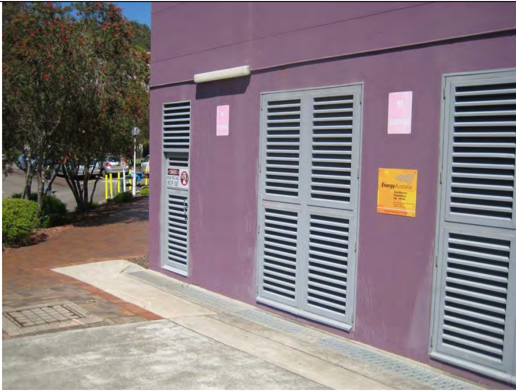
Photograph 3: The electrical substation located to the north of the site
