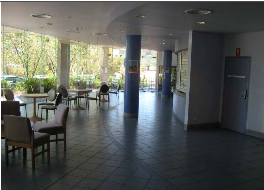
Photograph 6: The ground floor of the existing building. The ground floor currently consists of a former café, former reception area and offices
