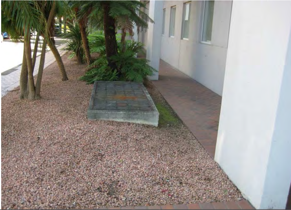
Photograph 7: The grease trap located along the southern boundary of the site. The grease trap was associated with the kitchen of the former café (shown above in Photograph 6)
