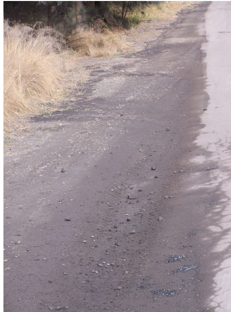
Figure 5 - Coal spillage on shoulder of Medway Road, Medway
