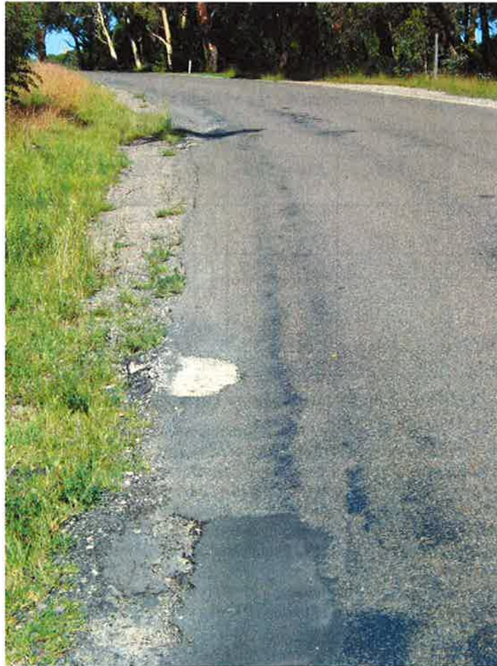
Figure 1 - Pavement failures on tight curve
