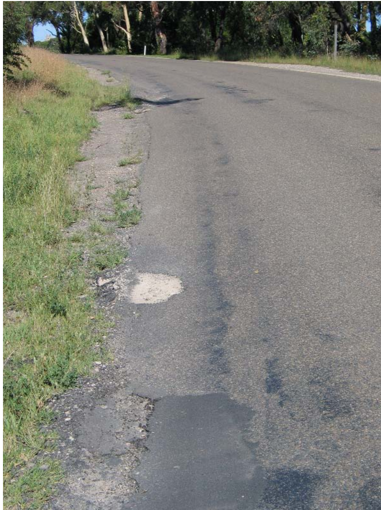
Figure 1 - Pavement failures on tight curve
