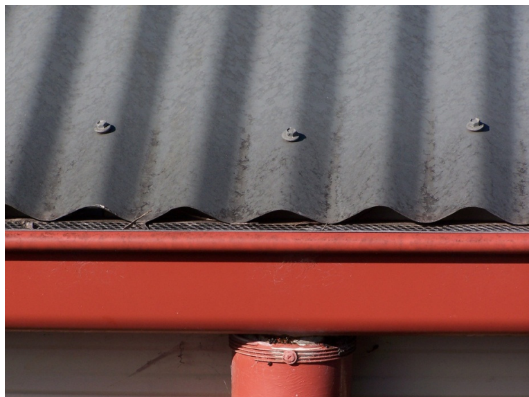
Figure 6 - Coal dust on houses and leading to water tanks
