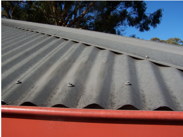
Figure 7 - Further view of coal dust accumulating on roofs
