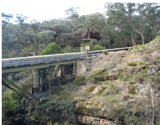
(a) Conveyor from mine to plant
