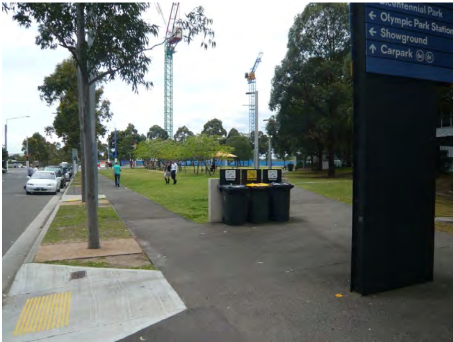
View looking east from Herb Elliott Avenue at the site for stage 1 of the development.
