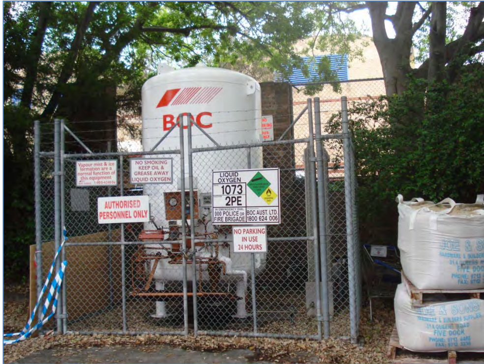
Plate P4: Oxygen tank in car park at rear of Building 21.
