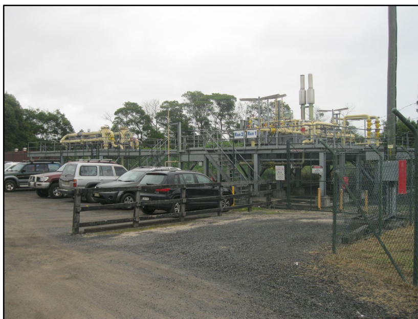
Plate 1: View of existing Gas Pressure Reduction Facility adjacent to CO 2 Plant.
