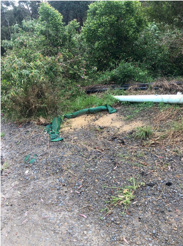
Photograph 19 – Improper use of erosion and sediment controls in areas that drains offsite
