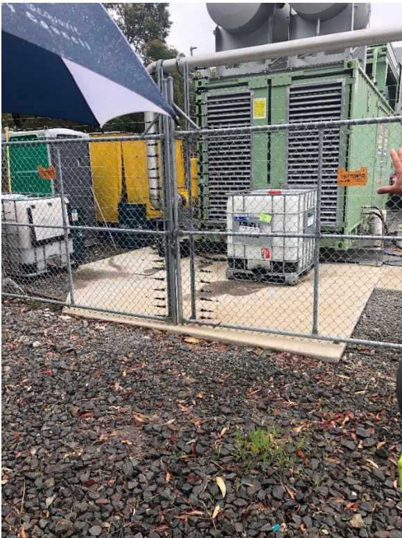
Photograph 12 – Gas energy plant at AWMF (hydrocarbon / chemical containers unbunded and leaking)
