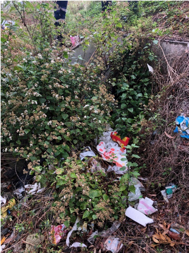
Photograph 09 – Weed growth and litter obstructing clean water diversion outlet
