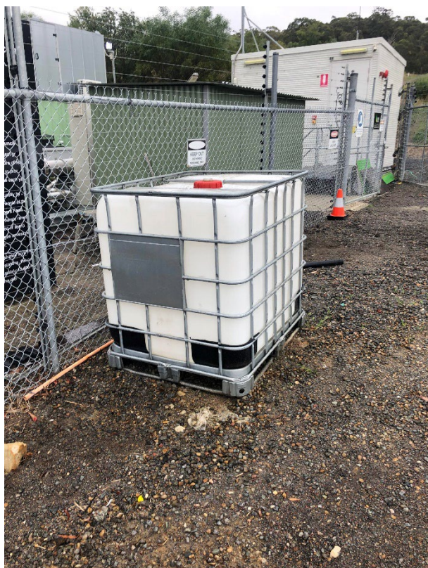
Photograph 13 - Fuels and chemicals were not located within bunded areas
