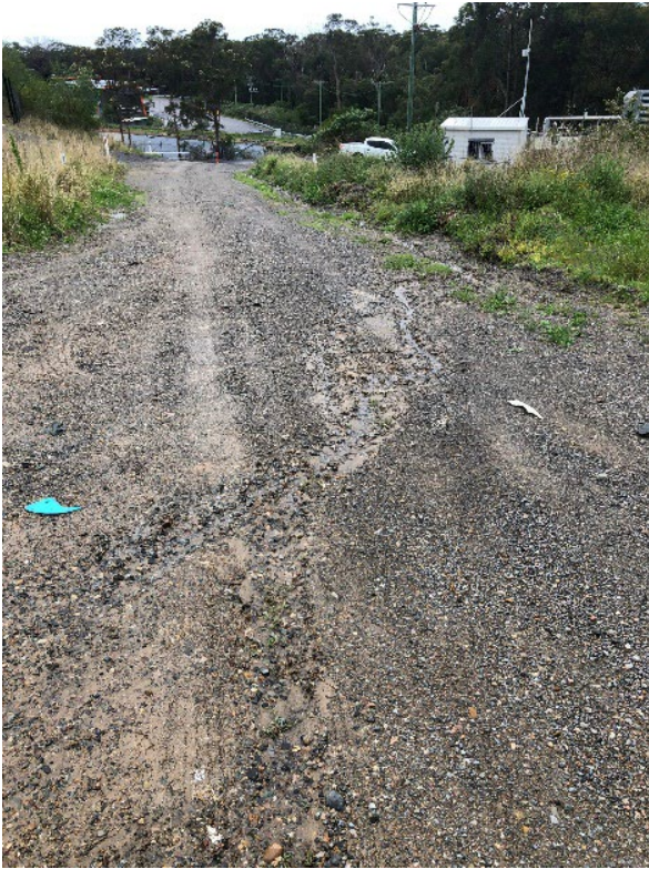
Photograph 17 – minor erosion of unsealed roads
