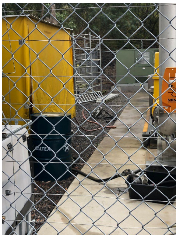
Photograph 14 – Hydrocarbon barrels located outside bunded areas
