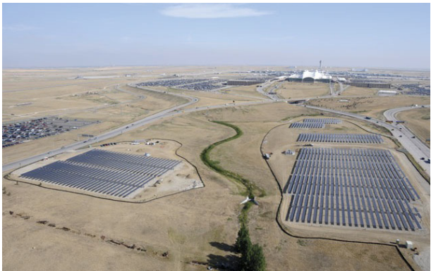
Denver International Airport Solar Farm http://www.oureverydayearth.com
