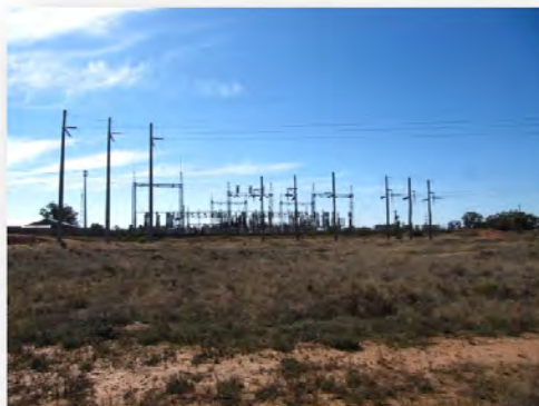
Photograph 26. Nyngan sub-station, south side.
