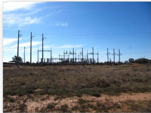
Photograph 26. Nyngan sub-station, south side.
