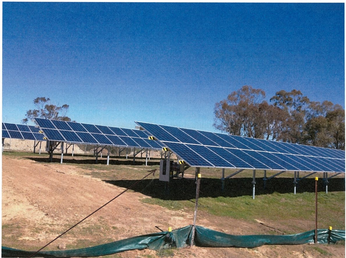
Figure 1. String Inverter mounted to a PV array frame.
