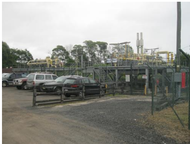
Image 2 – View of existing Gas Pressure Reduction Facility adjacent to the CO2 Plant
