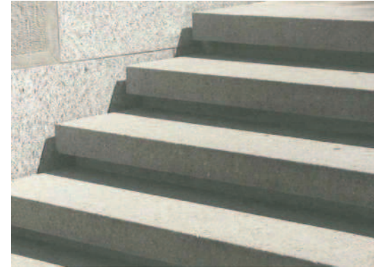
Step Type 1: Access stair 310mm wide x 155mm high treads granite to match paving
