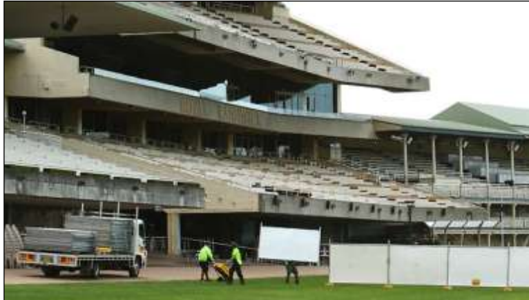
Figure 40: The collapsing upper level of the QE2 stand, photograph dated 1 st September 2011.
