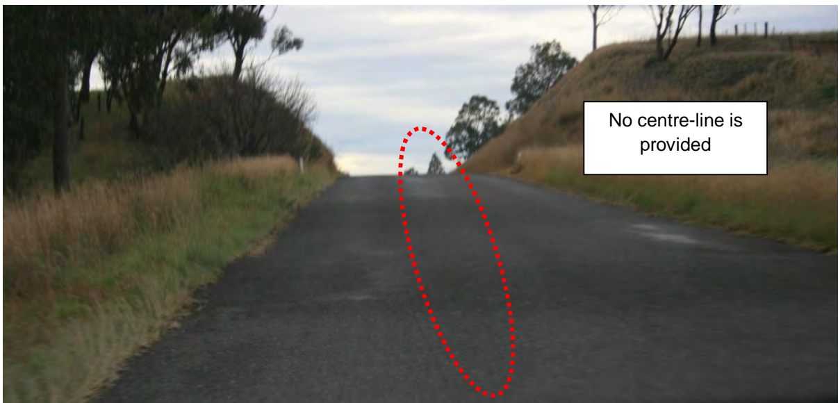
Photo 8 Bridgman Road, looking north towards the section to the south of Stoney Creek Road
