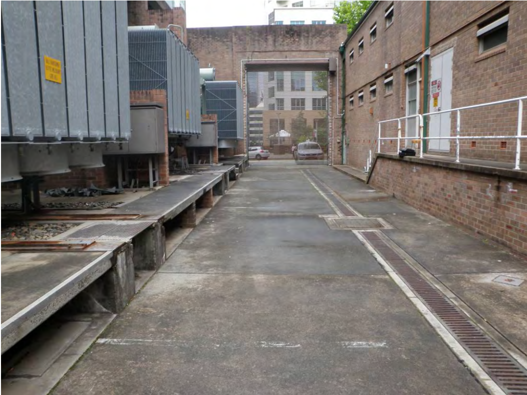
Plate P 1 Entrance to Substation
