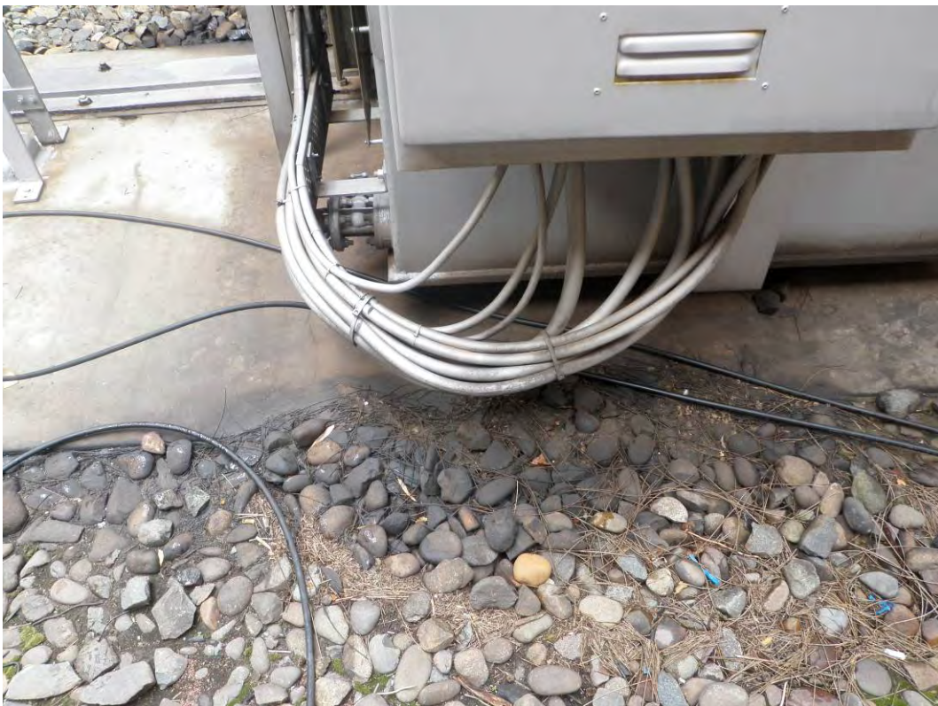
Plate P 4 Oil Staining beneath Transformer
