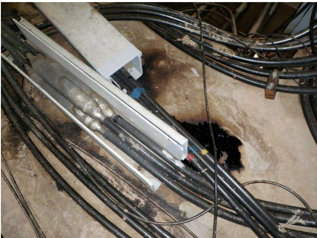
Plate P 2 Cable Room - Asbestos Boxing and Tar Leak
