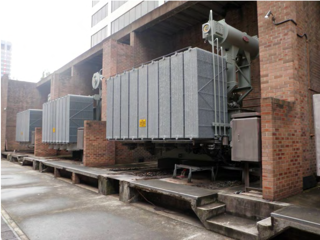
Plate P 3 Row of Transformers
