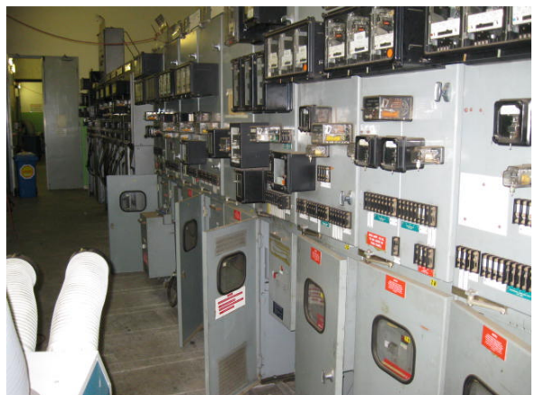
Plate 6: Electrical Equipment to 11KV Breaker Room presumed to contain ACMs.
