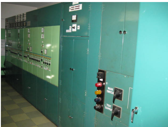
Plate 5: Electrical equipment within Battery Room presumed to contain ACMs.
