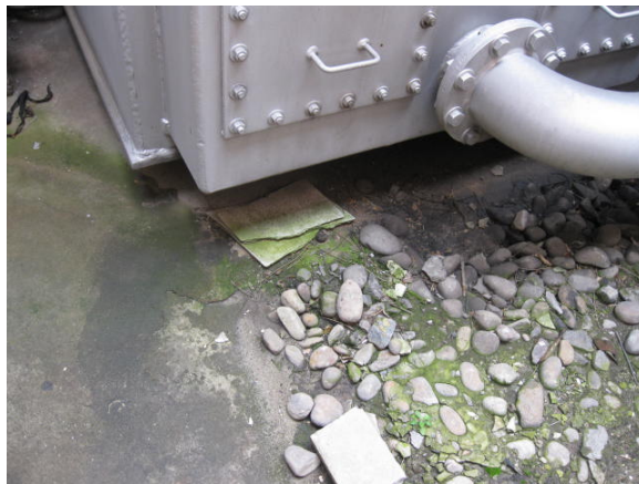
Plate 15: Possible PCB leaks indicated by staining to ground surfaces below transformers.
