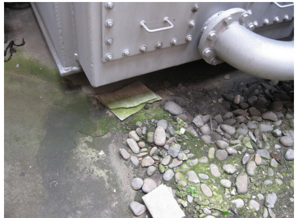
Plate 10: Fibre cement debris to the ground surface below Transformer 5 analysed and found not to contain asbestos.
