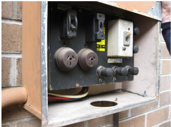
Plate 9: Asbestos containing backing board to Distribution Board MDB 69 located externally adjacent to Transformer 5.
