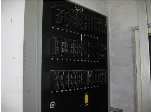
Plate 7: Distribution Board 1 (DB1) located in the Gas Room showing asbestos containing electrical backing board.
