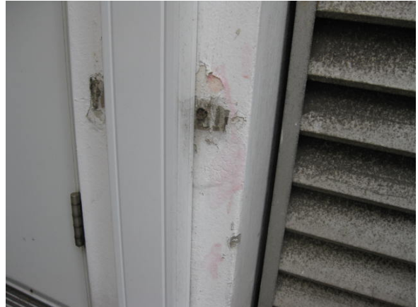
Plate 14: White lead paint to cement render adjacent to door of South West Plant Room.
