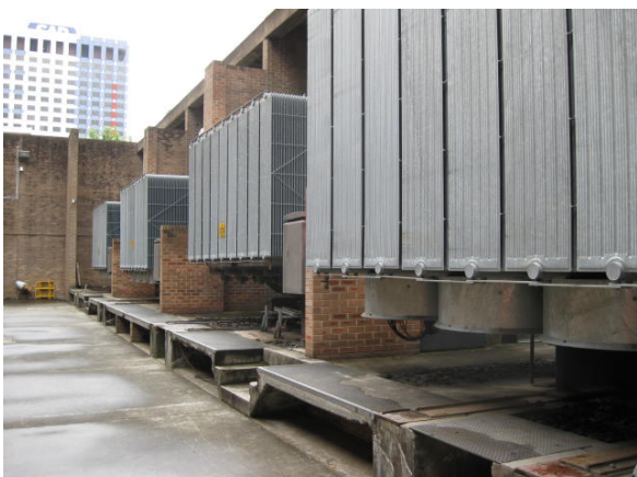
Plate 11: Transformers containing PCB insulating oil.
