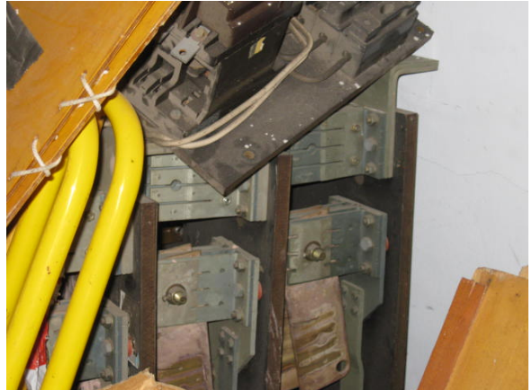
Plate 8: Redundant Electrical equipment containing asbestos cement spark shields and electrical backing boards located in the CLC Room,
