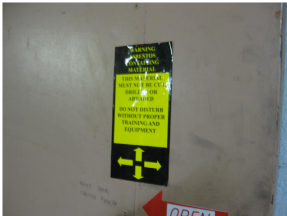
Plate 3: Typical Fire Door with presumed asbestos insulation core material.
