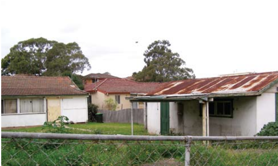
Figure 9 – Dilapidated buildings to the east of the site.
