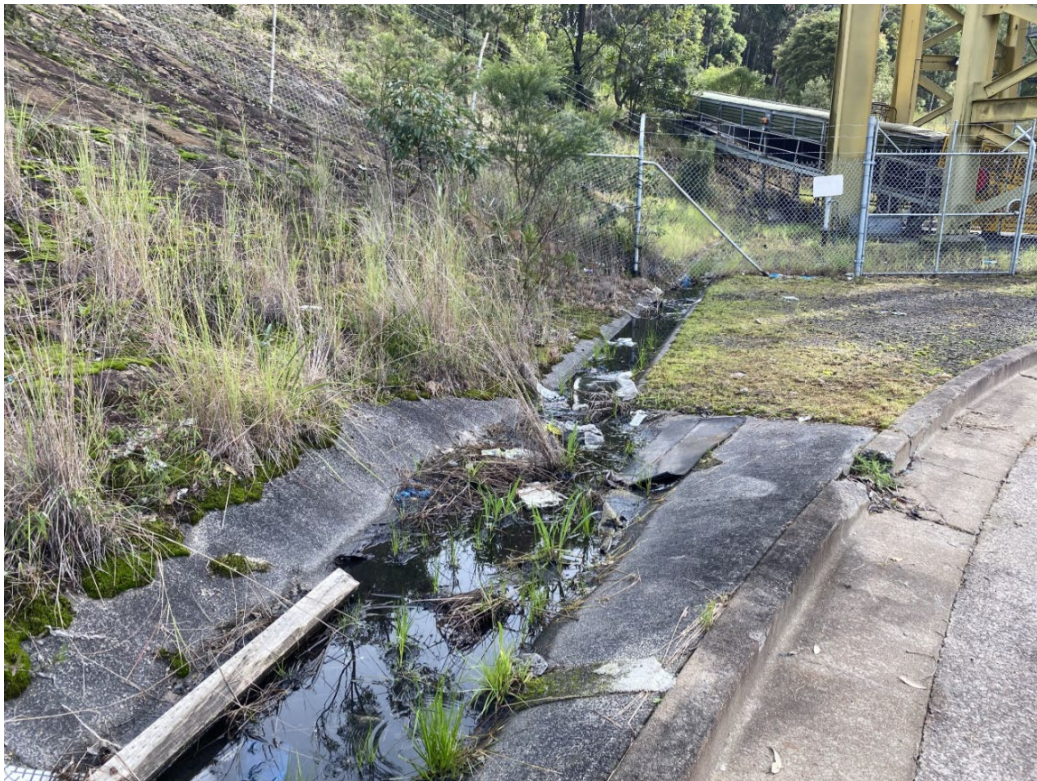
Photograph 30 – Waste in the clean water diversion drain down slope of the waste sorting area.
