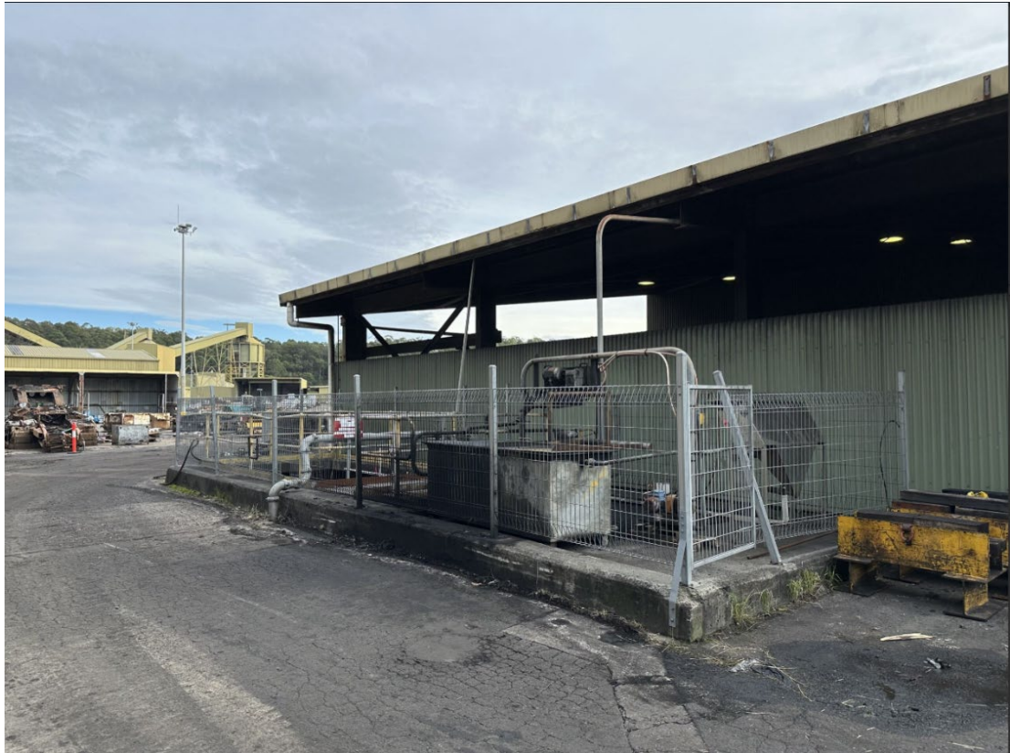
Photograph 09 – Oily water separator.
