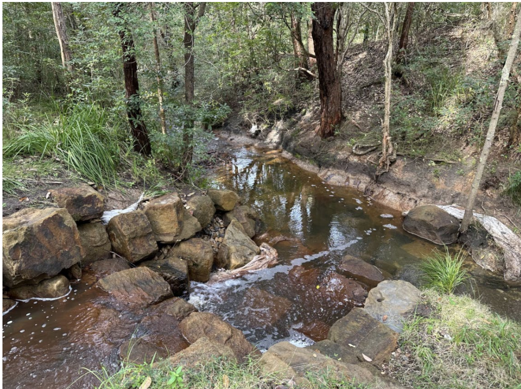
Photograph 42 – Wangi Creek remediation works. Note the unlodged bolder (see IMP REC 02).
