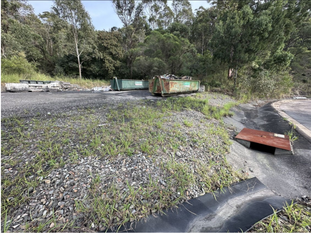
Photograph 29 – Clean water diversion drain down slope of the waste sorting area.
