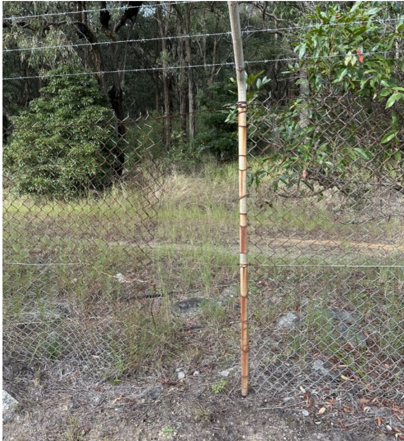
Photograph 25 – Damaged boundary fencing.
