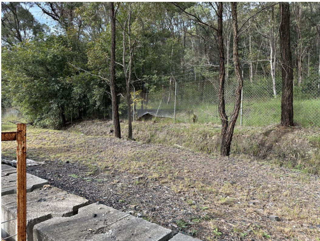
Photograph 24 – Damaged boundary fencing.
