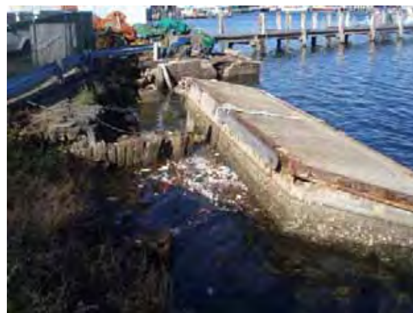
Concrete seawall in disrepair with relic timber structures behind
