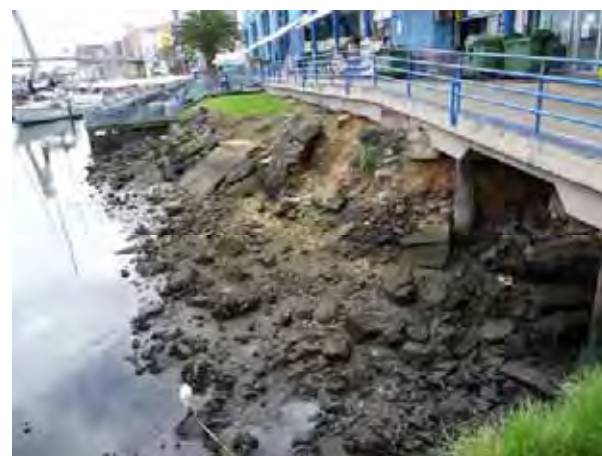
Rock edge seawall eroded from stormwater outlet with eroded rock bank stabilization required
