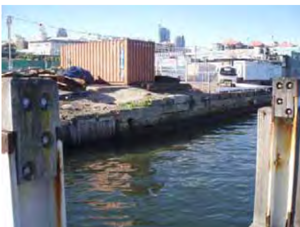
Sandstone seawall demarcating the original shoreline with seawall partially collapsed and subsided
