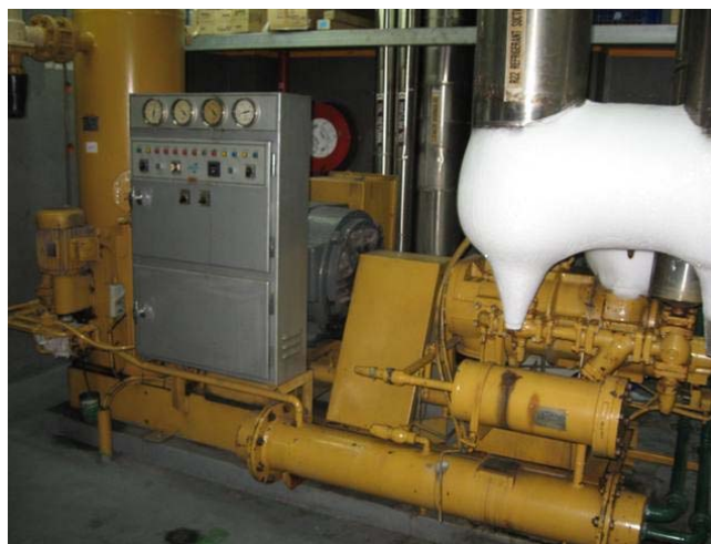
Existing R22 Compressor in Mezzanine Plant Room
