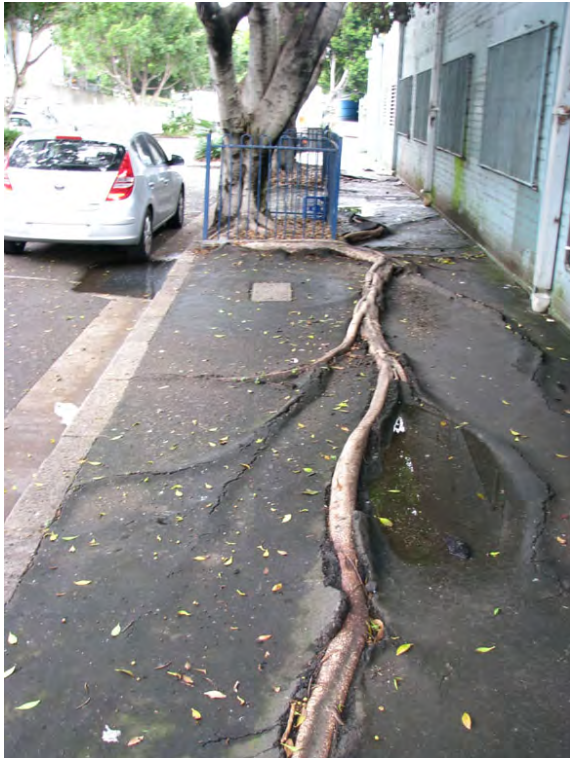
Figure 2: Hills Fig No. 20, together with 19 & 21, has continued to cause significant pavement damage
