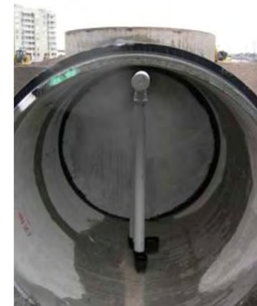
Underground stormwater tank
